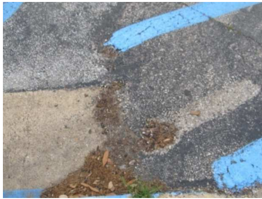
Figure 5-5 Rough patch near Tri-C parking lot - 3
