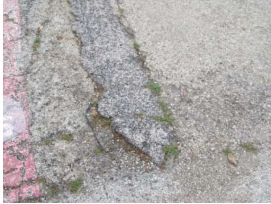
Figure 5-4 Rough patch near Tri-C parking lot - 2
