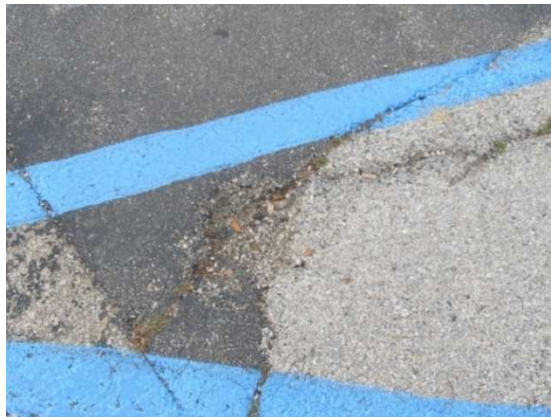
Figure 5-6 Rough patch near Tri-C parking lot - 4
