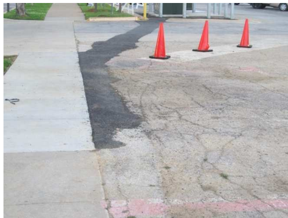
Figure 5-3 Rough patch near Tri-C parking lot - 1
