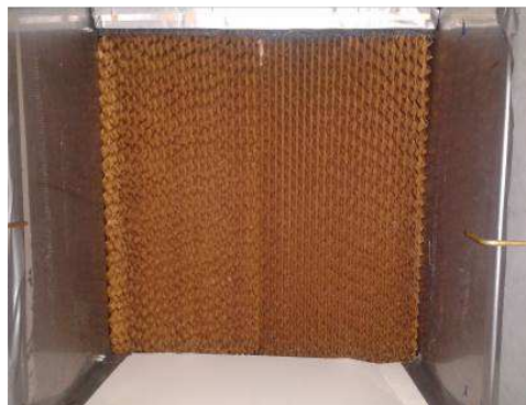
Figure 3.6: Rear view of the cooling pad (with both the pads fitted)
