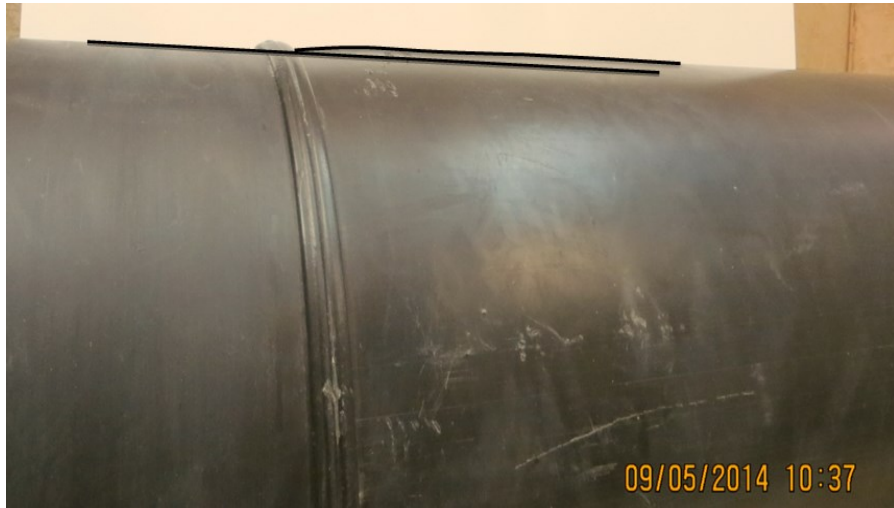
Figure 5.2 Pipe Bulge near Butt Joint
