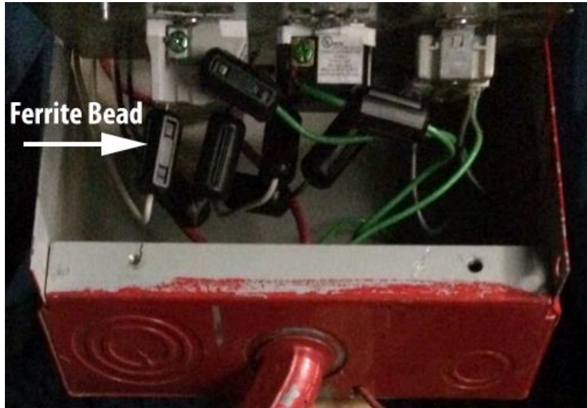
Figure 6-1 Ferrite beads placed on the hot, neutral, and earth ground lines of two brands of GFCIs. Note, the two ferrites on the hot line, though this proved to be unnecessary.
