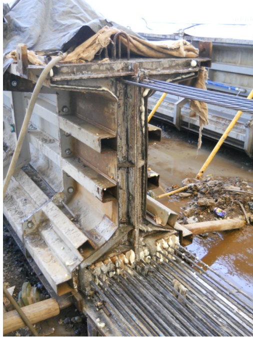
Figure 2.26: End girder view with wet mat for wet curing of the concrete.
