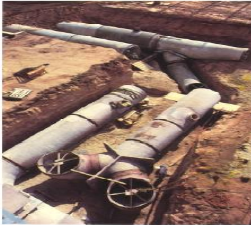
Special pipe sections and custom fittings are part of prestressing concrete cylinder pipe system at a power station (Ameron International).
