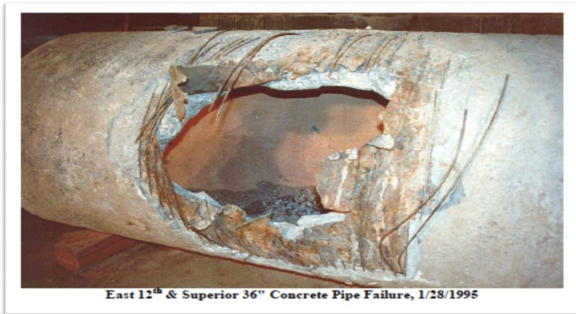
Figure 2.2 PCCP Rupture Failure due to Wire Break in 36-in. Diameter Size Pipe
