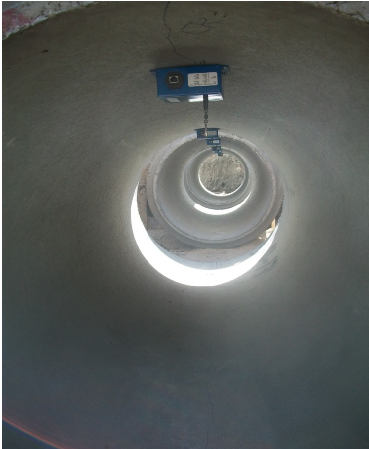
Figure A-17 Photograph of CDS device installed at crown
