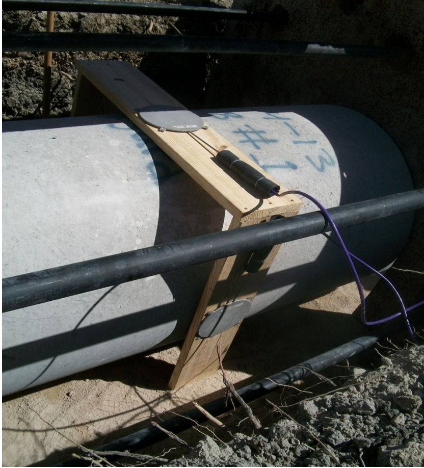
Figure A-18 Photograph of pressure transducer installed
