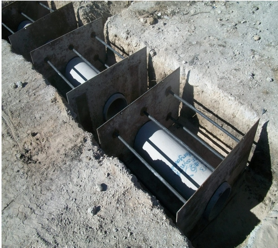
Figure A-16 Photograph of final set-up of steel capping for three pipes
