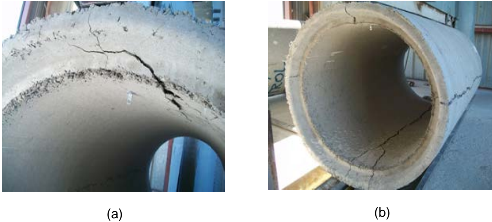
Figure 2-10 Cracks of 36 in. pipes; (a) regular reinforced pipe, (b) synthetic fiber reinforced pipe.
