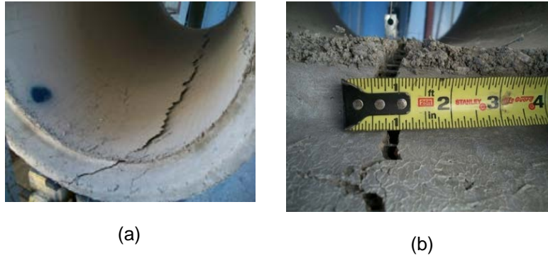
Figure 2-8 Main-crack at invert of 24. in pipes; (a) regular reinforced, (b) synthetic fiber reinforced
