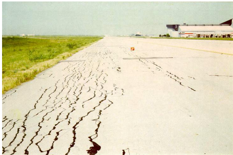
Figure 2-2 heave distress pattern on west shoulder of taxiway
