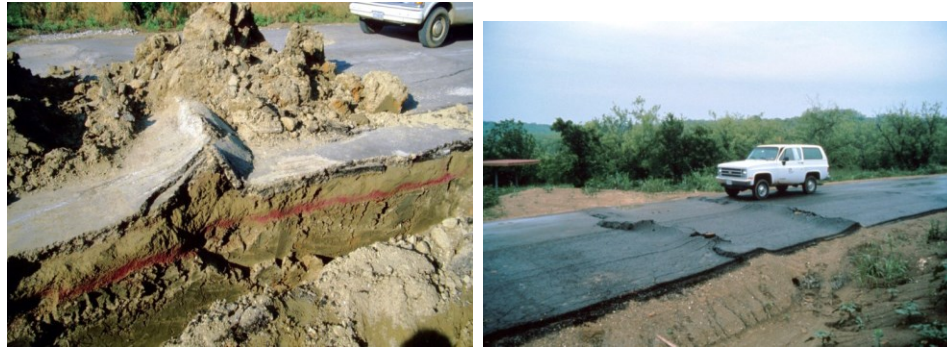
Figure 2-1 heaving in lime treated subgrade (Reproduced from Talluri, 2013)
