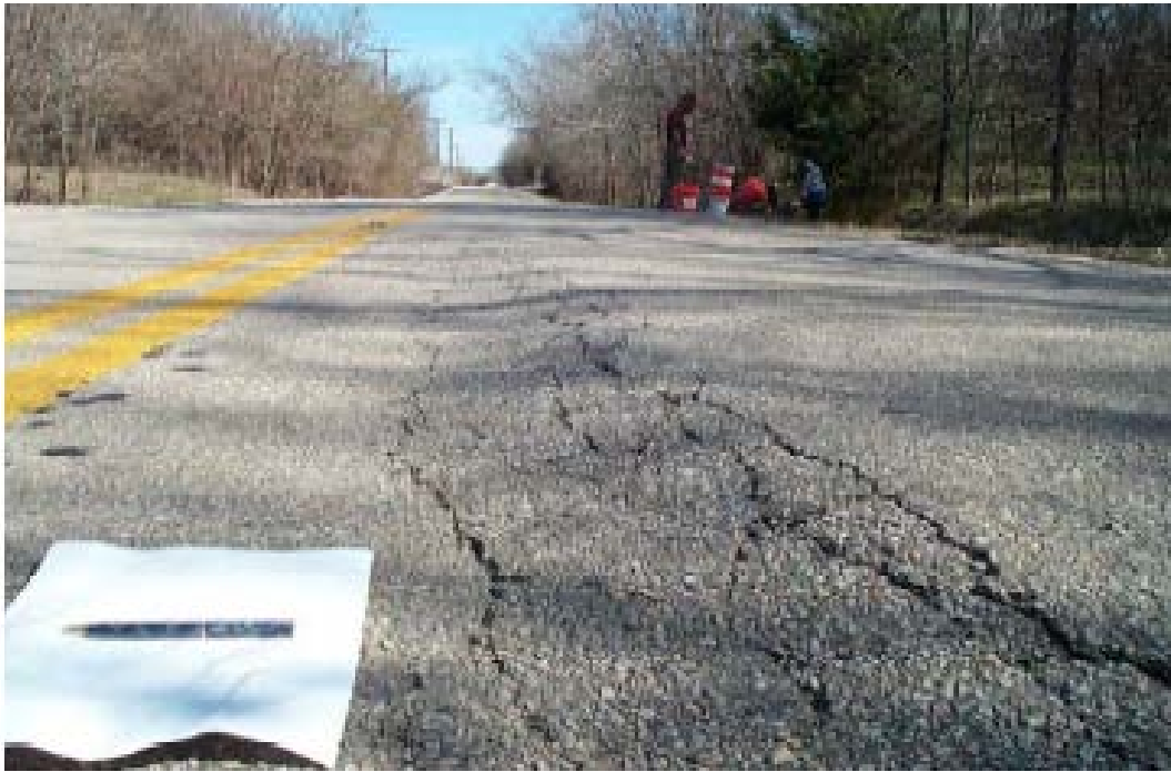
Figure 2-4 Pavement Distress Caused by Swell Shrink Phenomenon
