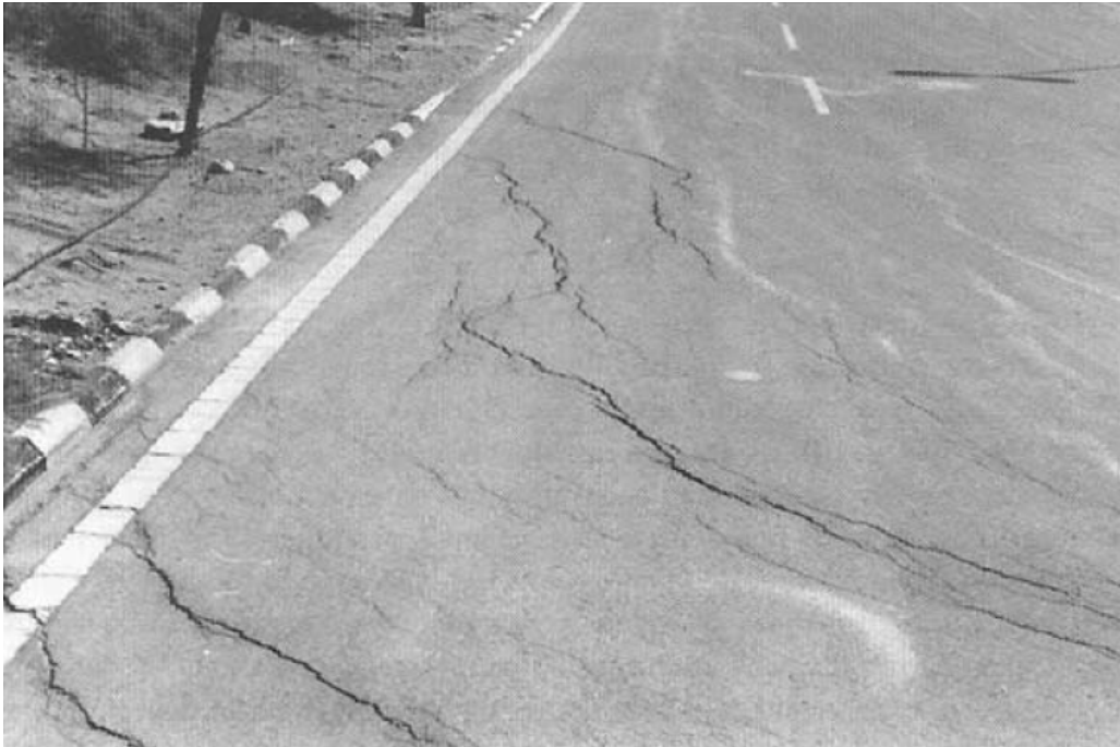
Figure 2-3 Pavement Failure (Al Rawas et al., 2005)
