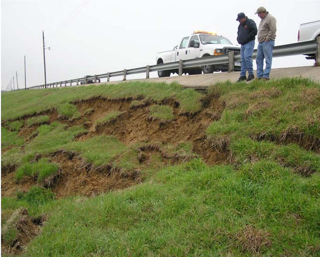
Figure 2-5 Slope Failure Triggered by Desiccation Cracks of Expansive Soils
