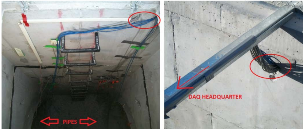
Figure 2 - 19 Concrete vault and cables path from the pipe to the DAQ headquarters
