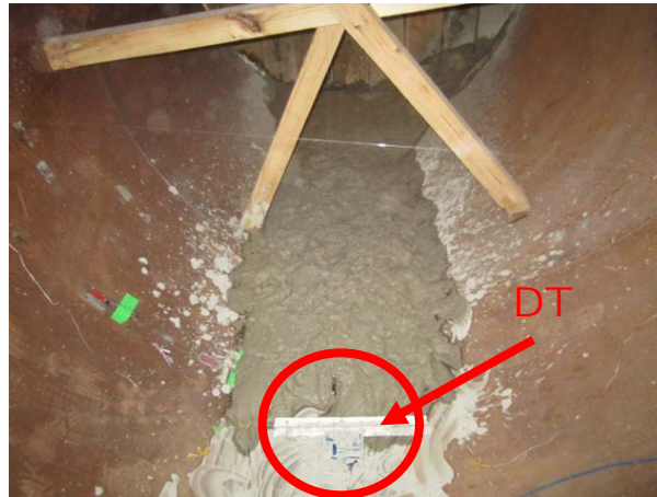
Figure 2 - 30 CLSM leaking inside pipe 1
