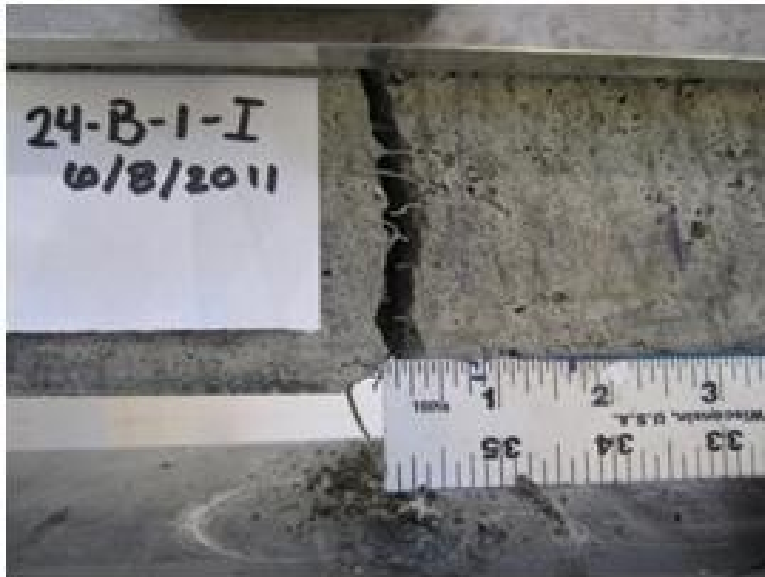
Figure D- 22 Crack pattern for NCP24-8-B-0.33-T2-BM
