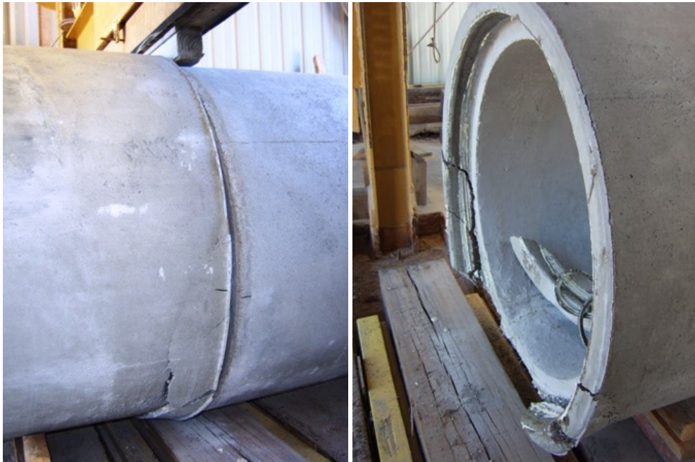
Figure B- 61 Specimen #2 joint shear failure pattern
