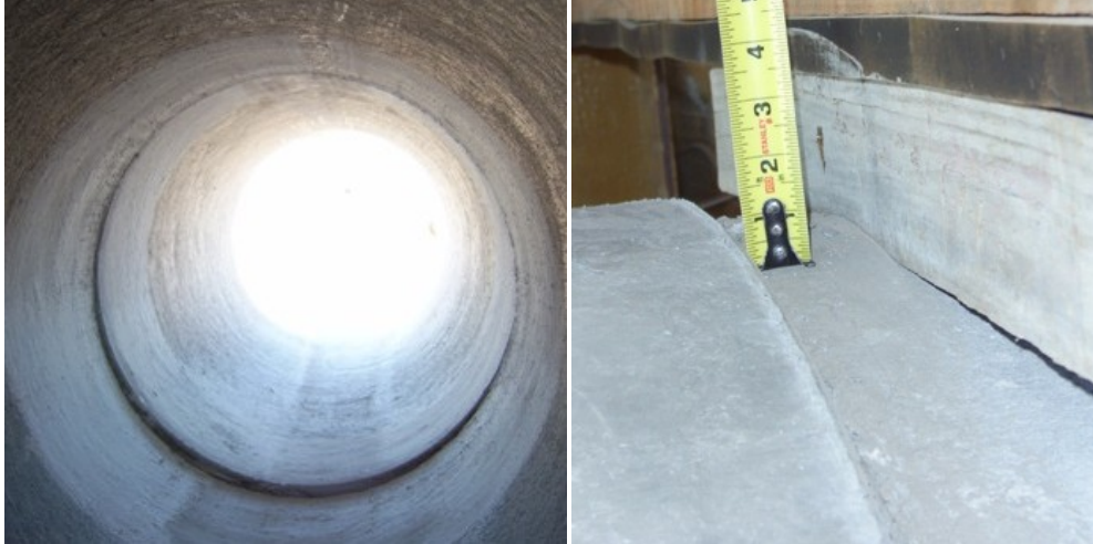
Figure B- 59 Specimen #1 joint shear differential failure
