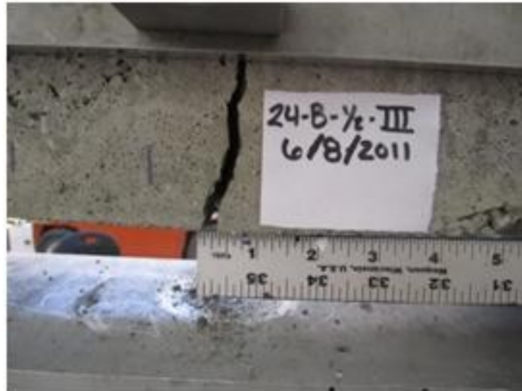
Figure D- 6 Crack pattern for NCP-24-B-0.17-T2
