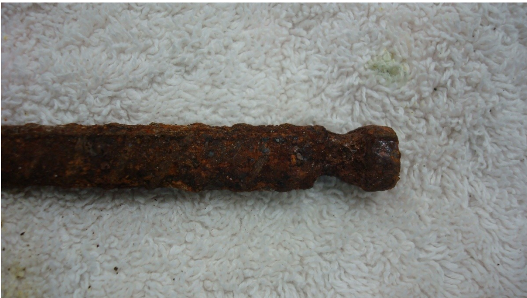
Figure 4-7 Rebar subjected to extreme localized corrosion
