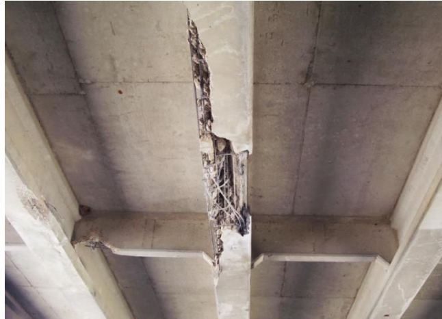
Figure 1-1 Damaged Concrete Girder
