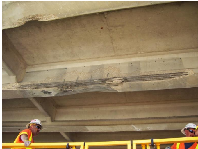
Figure 1-2 Wire Netting on the Bottom of Damaged Girder
