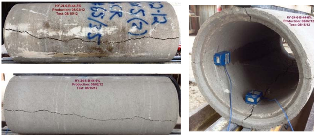
Figure B-20 Crack propagation for HYCP-24-6-B-44lbs steel-6%rubber
