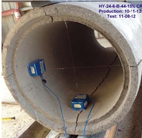
Figure 3-19 Photograph of crack failure mode in 24 and 36 in. pipes
