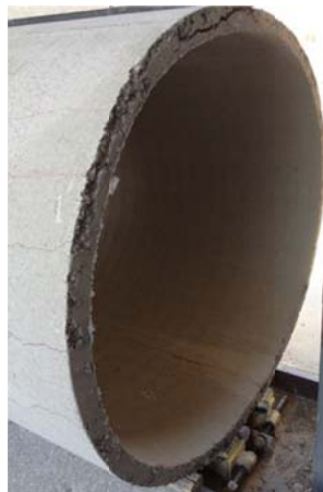
Figure 3-20 Photograph of crack failure mode in 54 and 60 in. pipes
