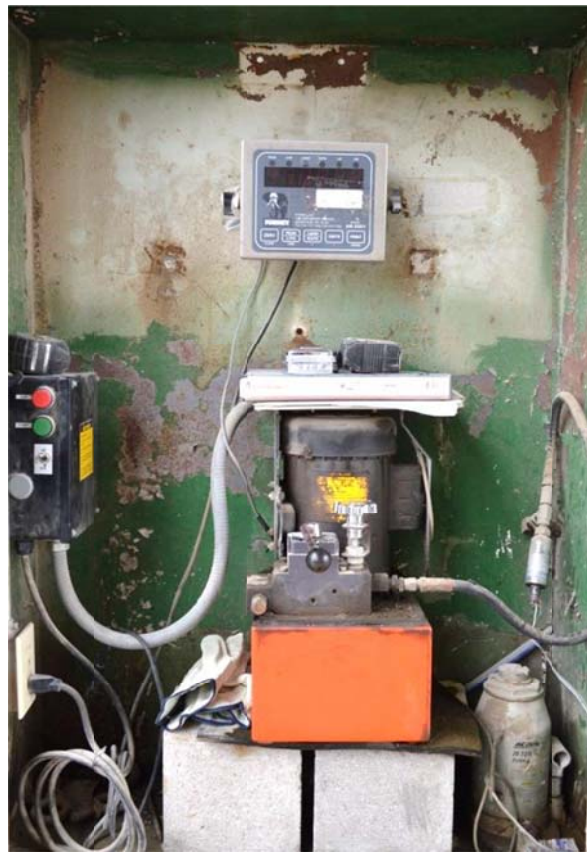
Figure 3-4 Photograph of load cell at Hanson facility
