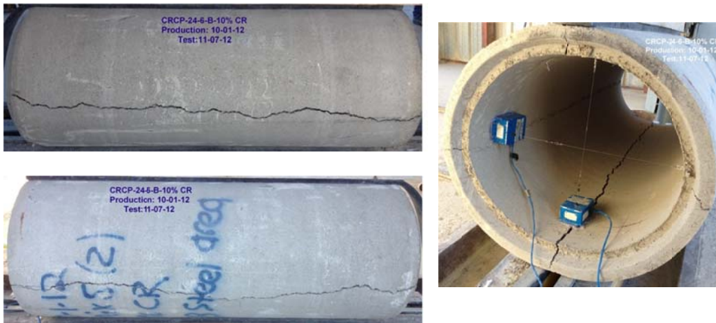
Figure B-88 Crack propagation for CRCP-24-6-B-10%rubber
