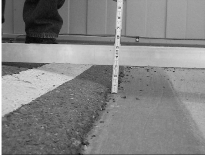
Figure 2.9 Heaving in flexible pavement near northeast corner of hangar
