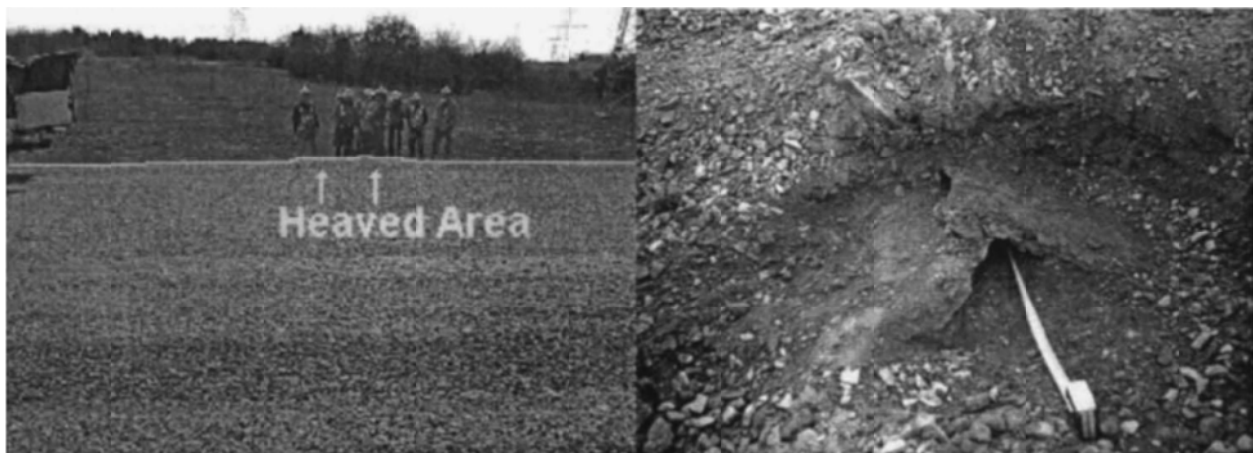
Figure 2.13 Heaved area on east bound side
