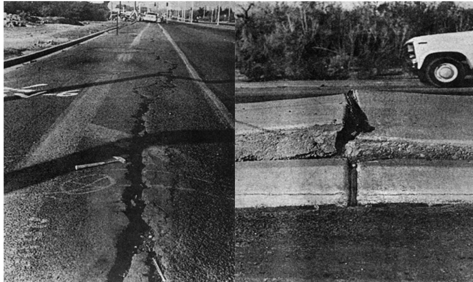
Figure 2.7 Longitudinal and Transverse cracks on Stewart Avenue (Hunter, 1988)
