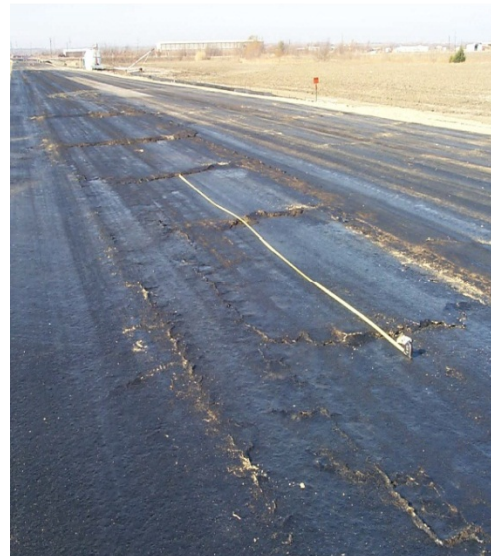
Figure 2.1 Severe Pavement Distress along US 67, Texas
