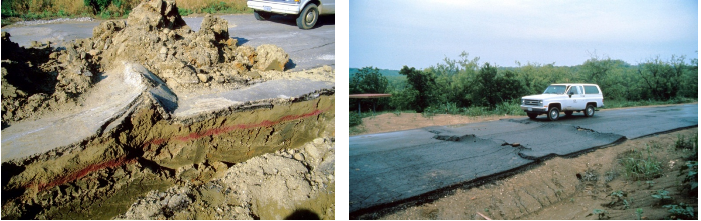
Figure 2.10 Heaving in lime treated subgrade
