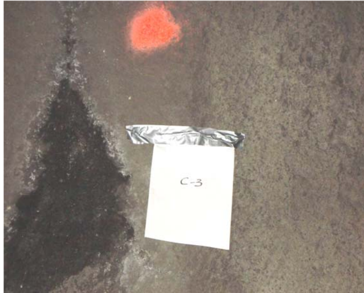
Figure 2.11 Distress region on tunnel lining (C-3)
