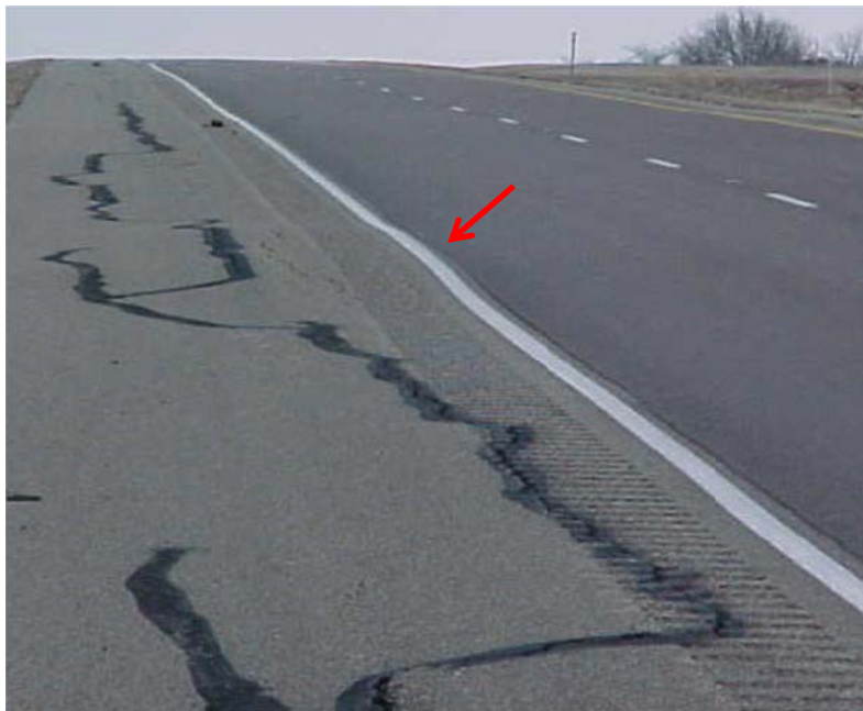
Figure 2.14 Longitudinal Cracks on Shoulder and Swell
