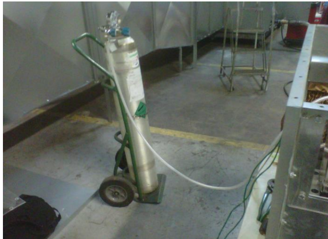
Figure 5.10 Cylinder safely strapped to ensure safety
