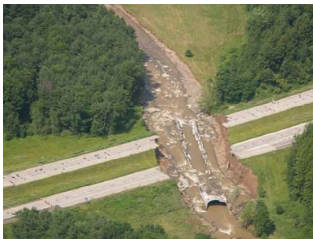
Figure 1-1 Culvert Failure on Interstate-88 June, 2006 (FHWA, 2007)
