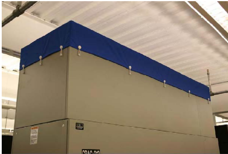
Figure 5.16 The Covering of the CRAH Units [122].
