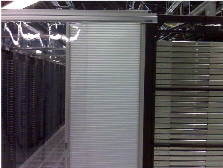
Figure 5.7 The Cold Aisle Containment System.
