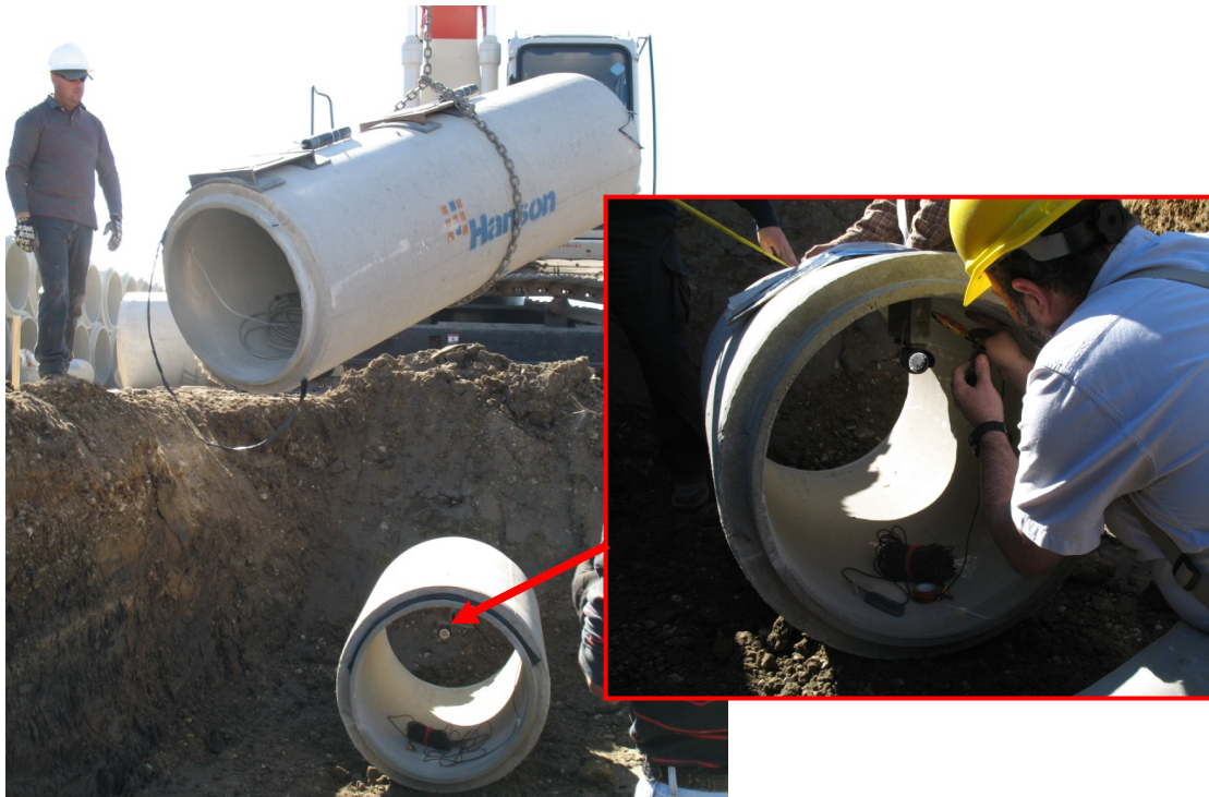
Figure 2.10 an installed inspection camera at a supporting pipe.
