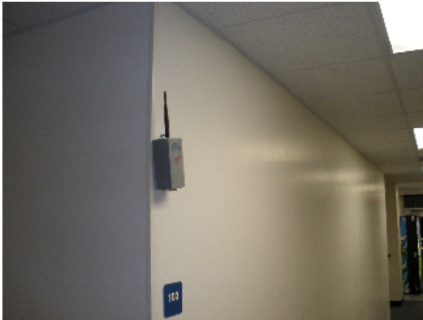
Figure 7.3. An accesspoint installed on the wall.
