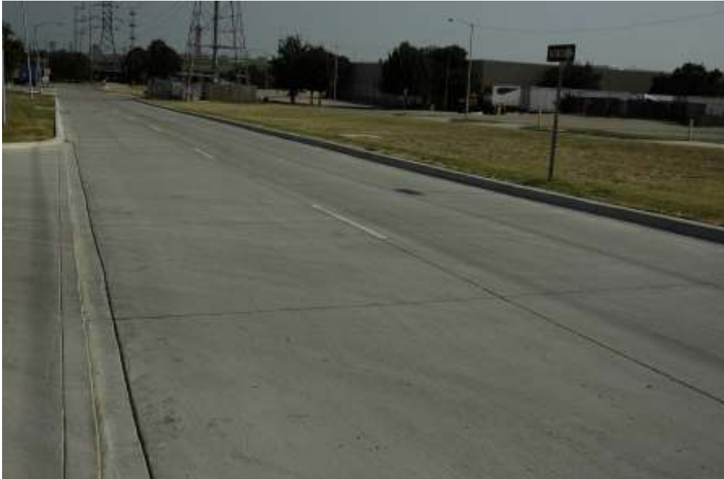
Figure 6.30 Current Condition of Pavement at International Parkway (30 Months after Reconstruction).
