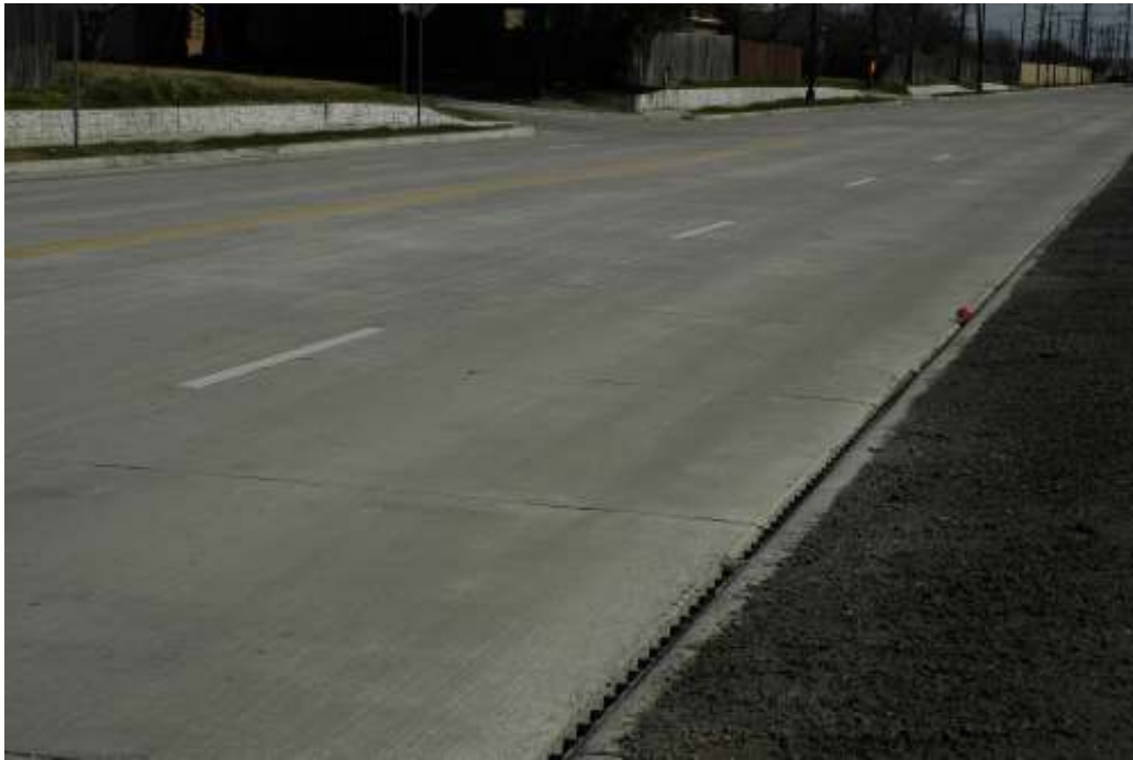
Figure 6.45 Current Condition of Southmoor Drive (Continue).
