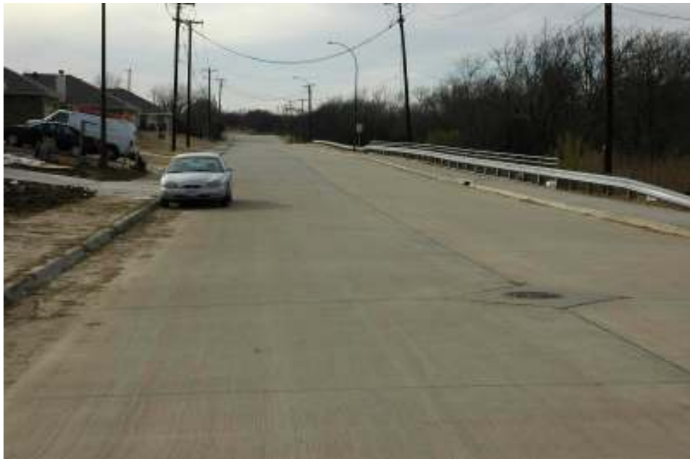
Figure A4 Current Condition of Harwood Road (Lime with Fibers Treated Section).
