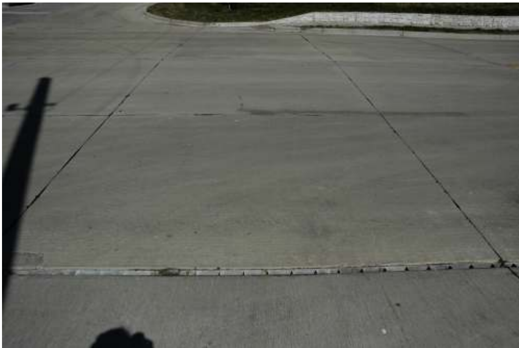
Figure 6.44 Current Condition of Southmoor Drive (Continue).
