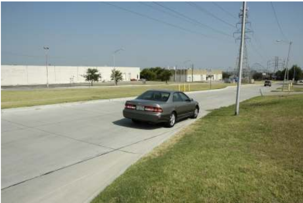
Figure 6.31 Current Condition of Pavement at International Parkway (Continue).
