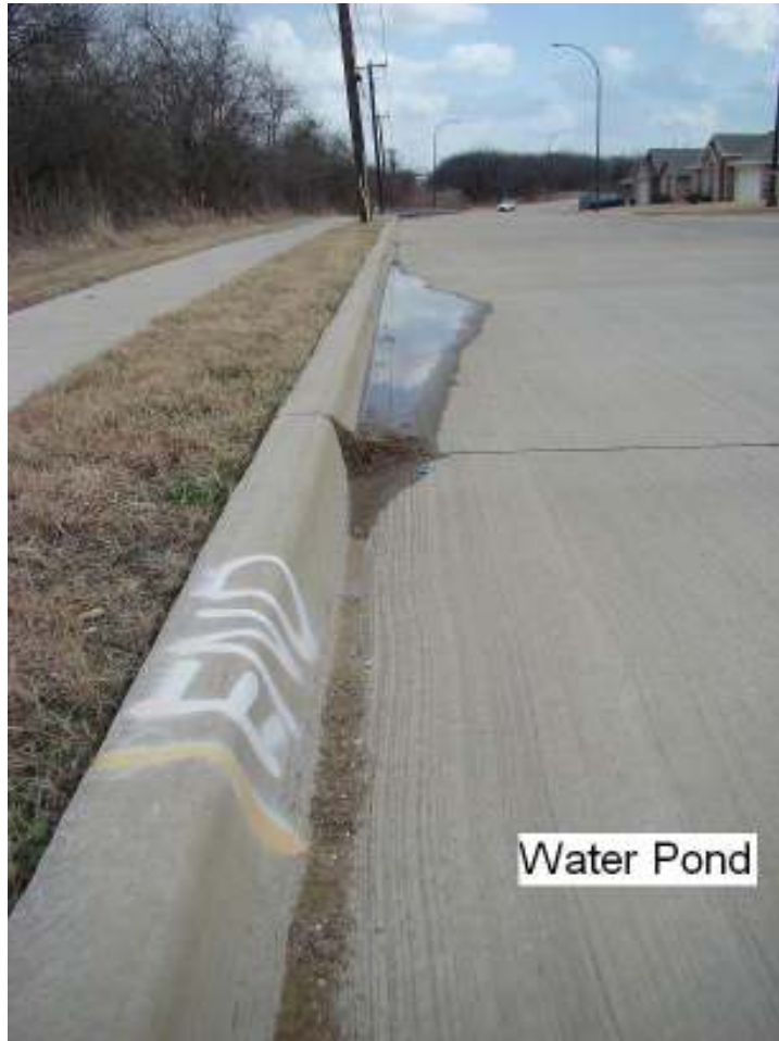
Figure 6.25 Water accumulation on pavement at control (lime treated) section.
