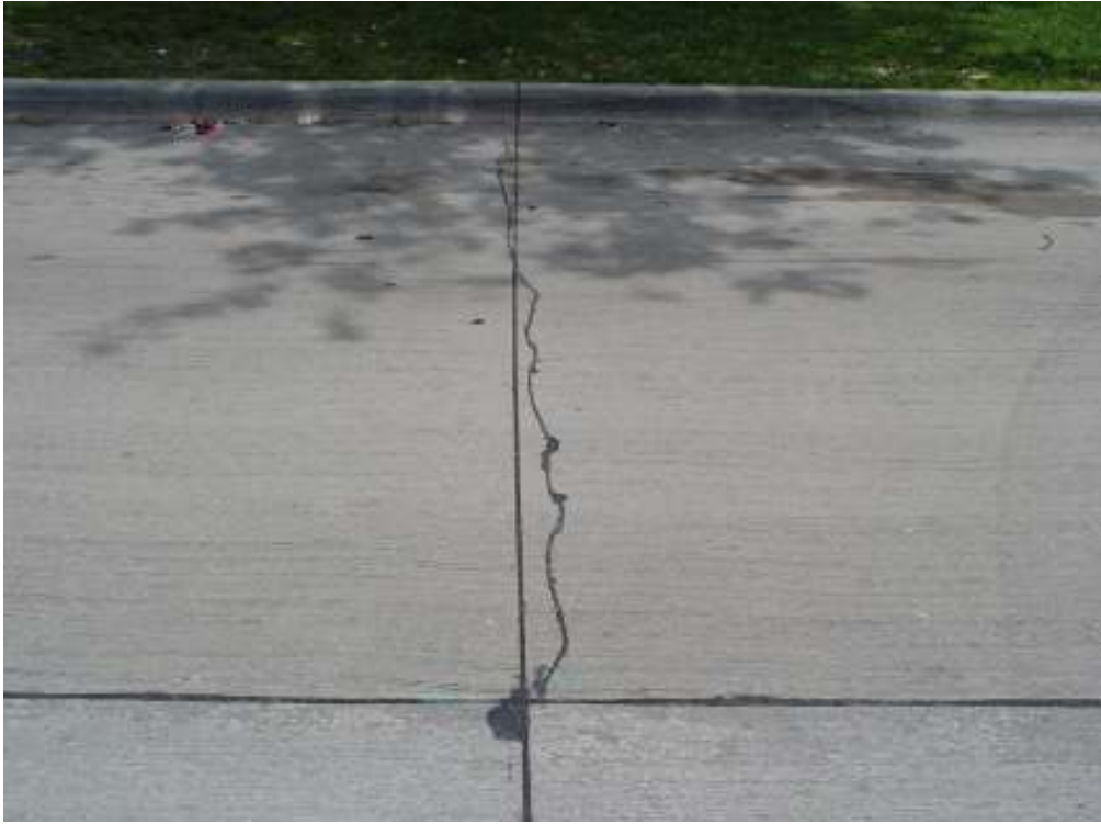
Figure 6.38 A Hairline Crack Observed on the Paved Area of Southmoor Drive.
