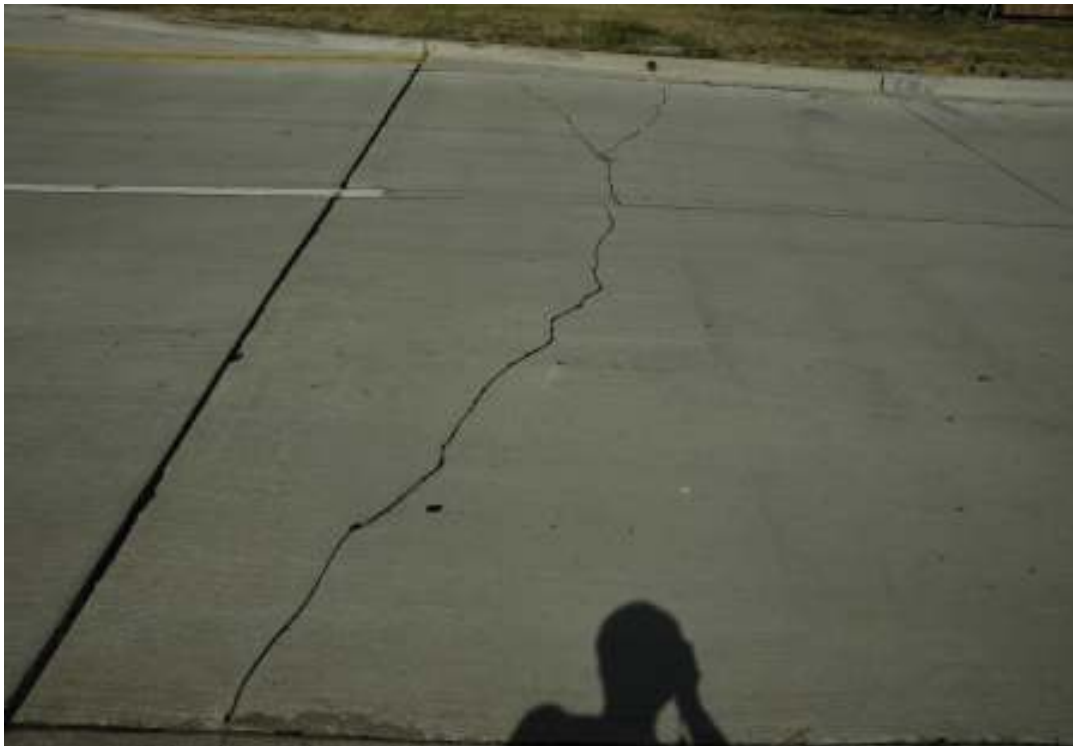
Figure 6.33 Hair Line Crack Observed at International Parkway.
