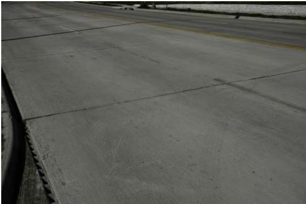
Figure 6.42 Current Condition of Southmoor Drive.
