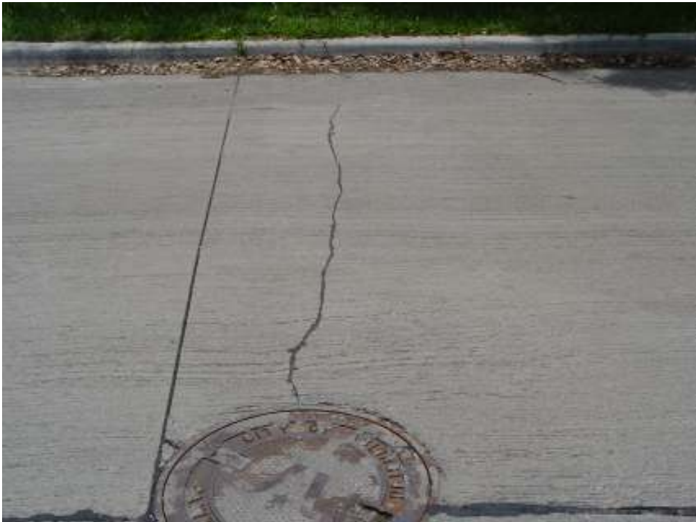
Figure 6.39 A Hairline Crack Observed at Near The Manhole, Southmoor Drive.
