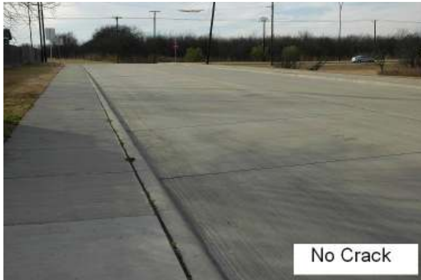
Figure 6.21 Condition of pavement at section 1 (Type V Cement stabilized) after 39 months.
