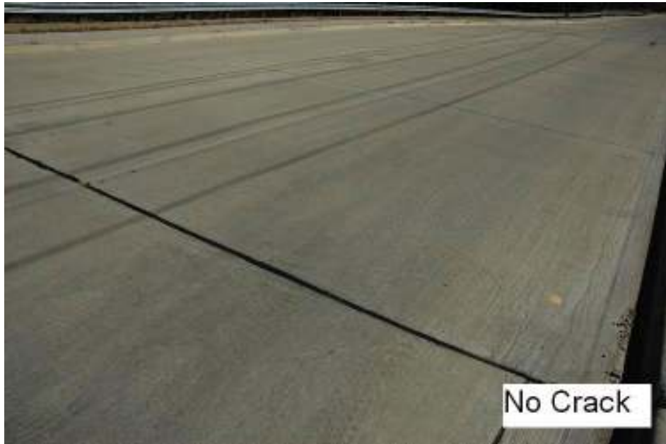
Figure 6.24 Condition of Pavement at Section 4 (Lime and Fiber stabilized Subgrade) After 39 Months.
