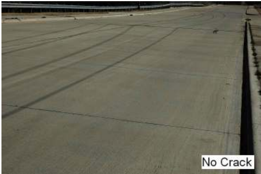
Figure 6.23 Condition of pavement at section 3 (GGBFS stabilized) after 39 months.
