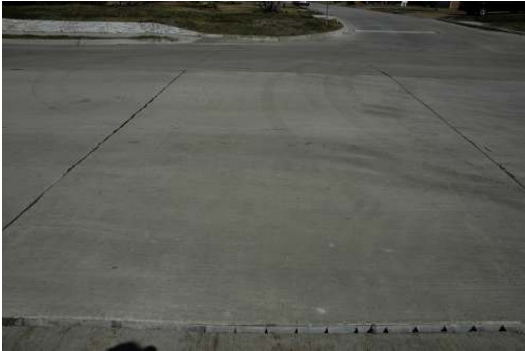
Figure 6.43 Current Condition of Southmoor Drive (Continue).
