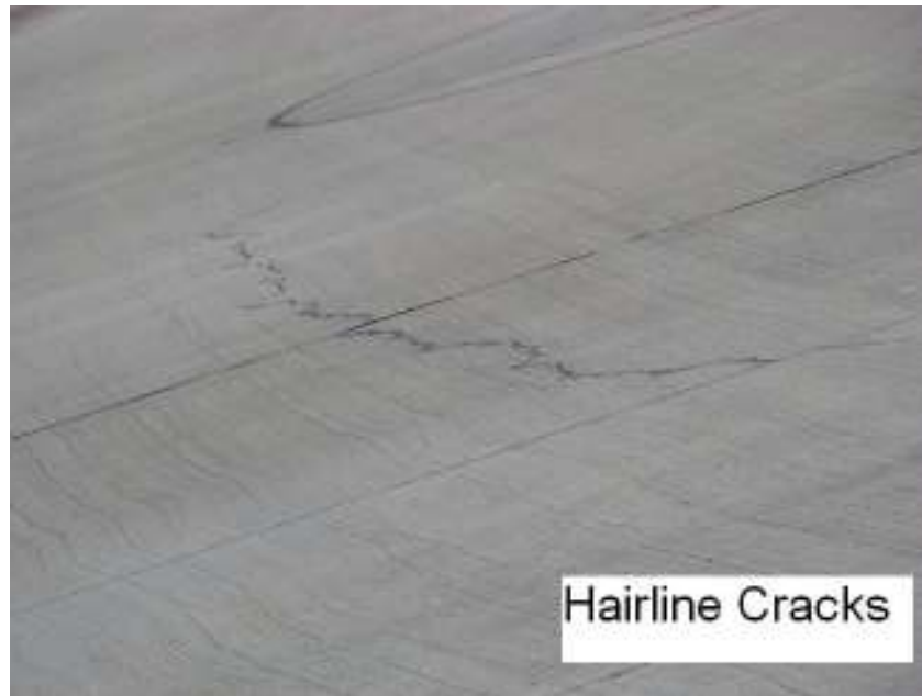
Figure 6.26 Longitudinal and Transverse cracks observed at control section.
