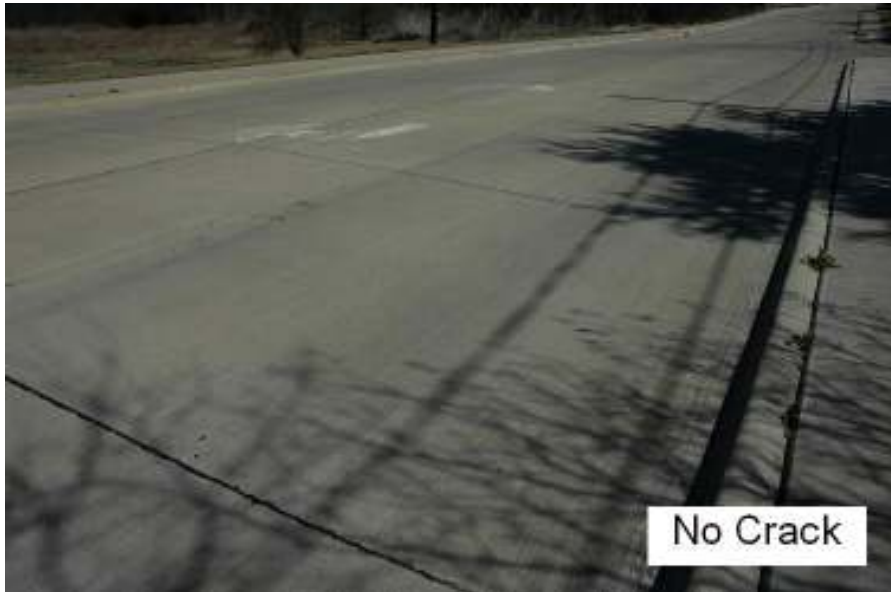
Figure 6.22 Condition of pavement at section 2 (Cement and Fly ash stabilized) after 39 months.
