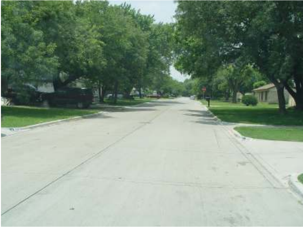
Figure 6.36 Current Condition of Southmoor Drive.
