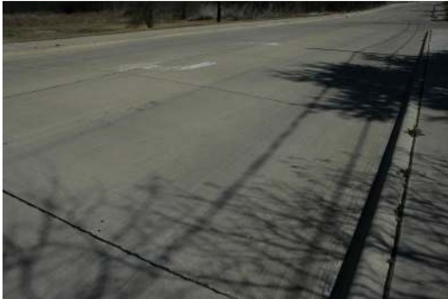
Figure A2 Current Condition of Harwood Road (Cement with Fly ash Treated Section).
