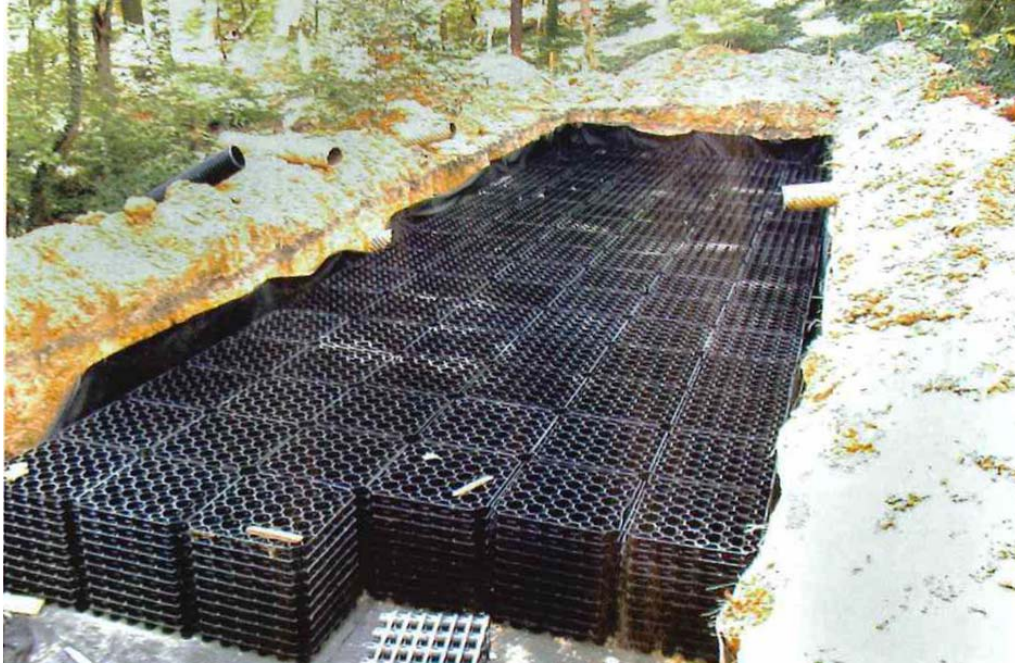
Figure 2.24: Infiltration basin at Olmsted Woods at the Washington National Cathedral during construction (McIntyre, 2006a)
