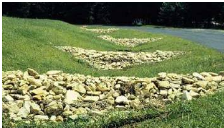
Figure 2.21: Roadside dry grass swale containing rock check dams within a residential area (Lake Superior Streams, 2005)
