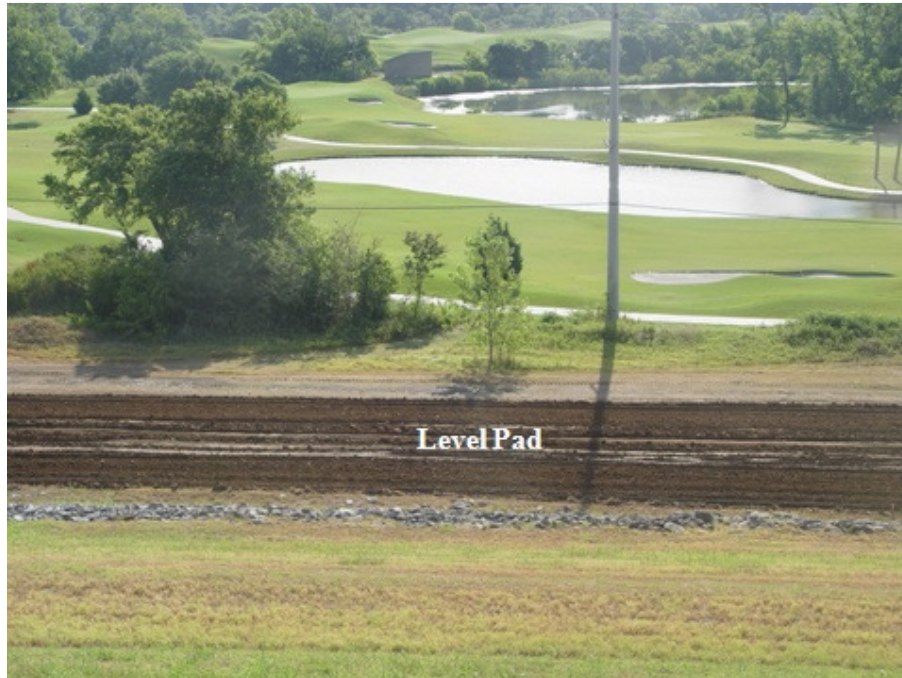
Figure 4.12 Pulverized and moistened soil at level pad ready for mixing with admixtures
