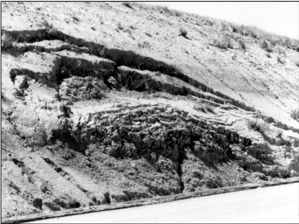
Figure 2.2 Surficial failure triggered by heavy rains in Colorado in 1973 (Source: USGS)
