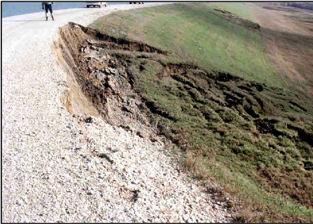
Figure 1.1 Surficial failure at Bardwell Dam (Source: USACE)
