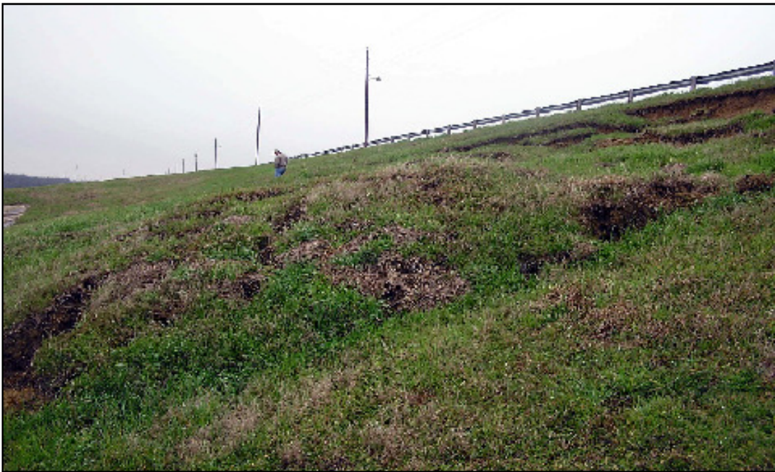
Figure 2.11 A Surficial slope failure at the Grapevine Dam, Texas, USA
