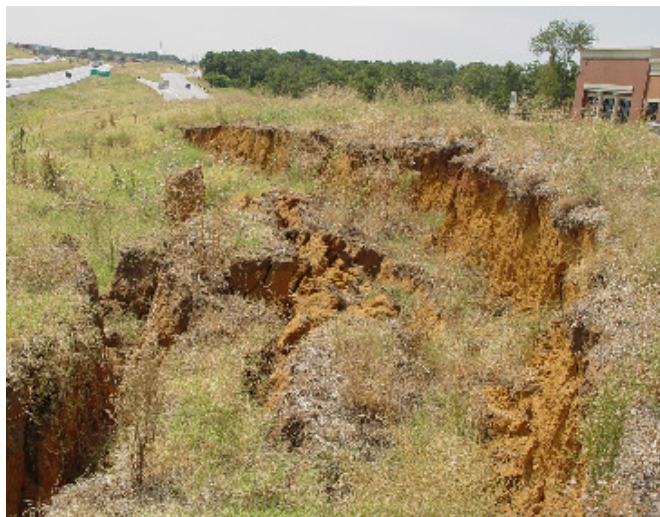
Figure 2.12 Surficial failure of a cut slope on SH 360 near the DFW airport, Texas
