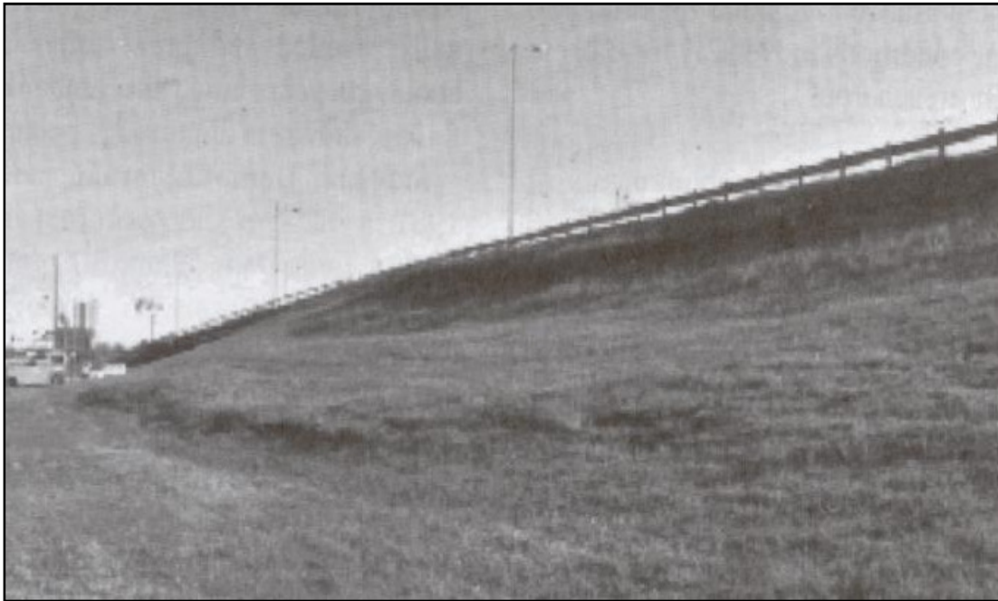
Figure 2.24 A surficial slide near Houston on highway embankment (Source: Duncan and Wright, 2005)
