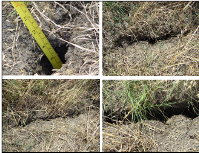
Figure 5.35 Cracks near construction joint of control and compost sections
