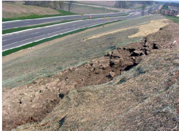
Figure 2.38 Surficial failure on a cut slope along STH-164, Wisconsin (Source: Titi and Helwany, 2007)
