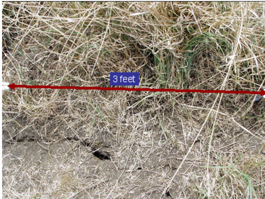
Figure 5.36 Digital image of cracked surface in control section
