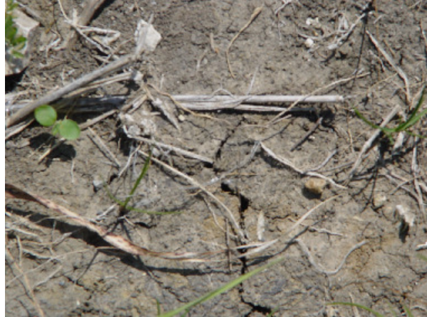
Figure 5.32 Minor cracks noticed during March 2008 at Joe Pool Dam
