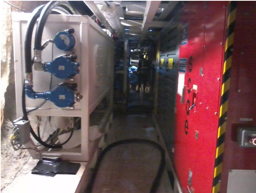
Transformers and hydraulics located on the TBM trailing gear.
