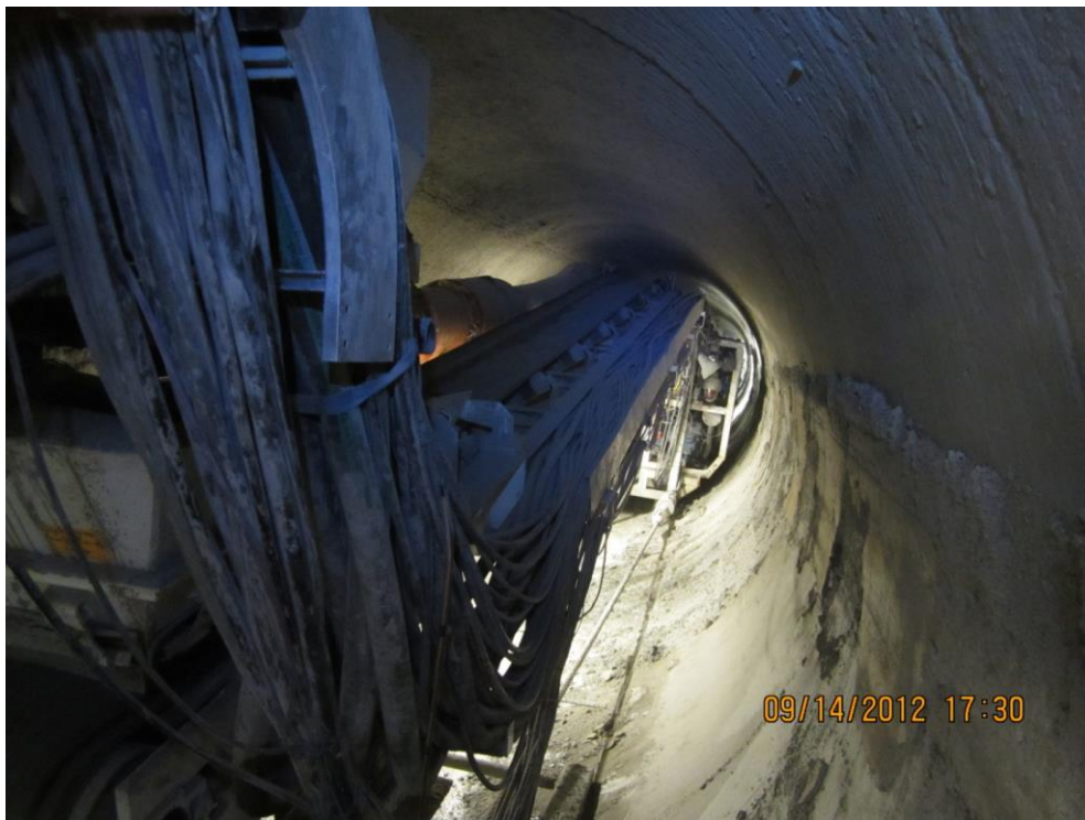
View from the back of the operator's cab towards the trailing gear.
