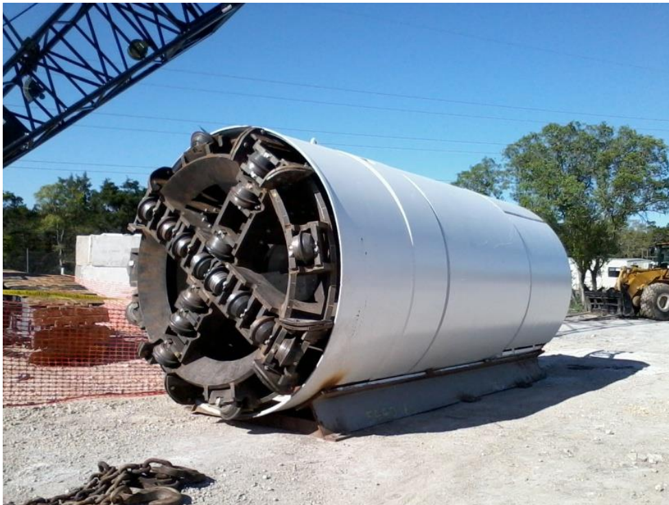
Figure 1.3. Cutter head and TBM can, which will hold the TBM operator and contains the grippers. This particular cutter head was built by Southland Contracting and used on Reach #1 of the Jollyville Transmission Main project in Austin, Texas.
