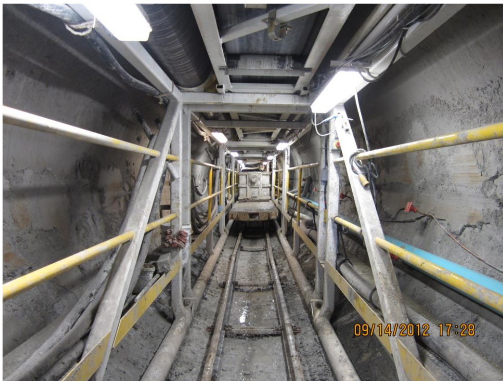
The back-up system with a muck car being pushed under the conveyor system.
