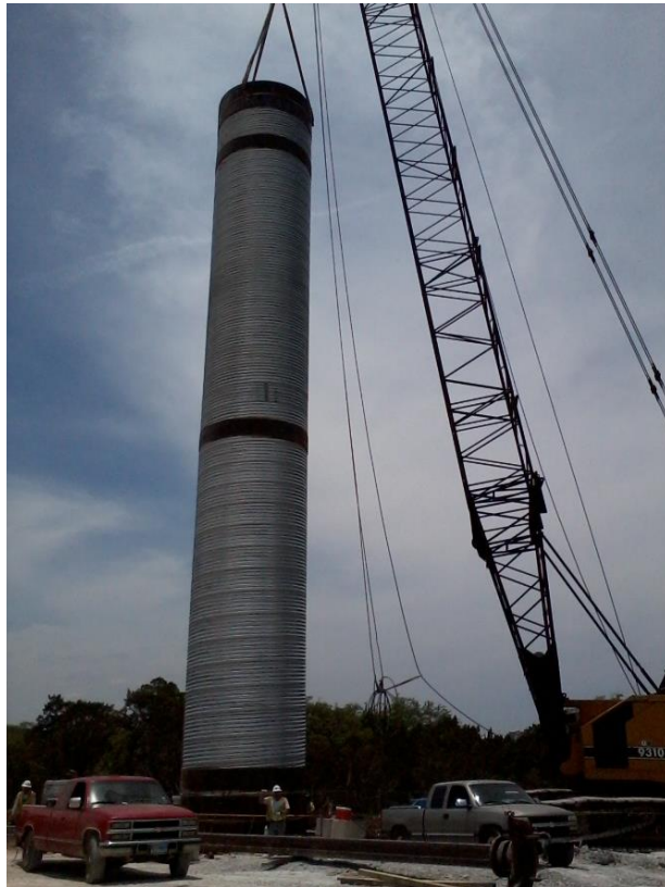
Figure 1.12. The steel casing being lowered into the shaft at the WTP4 shaft site.
