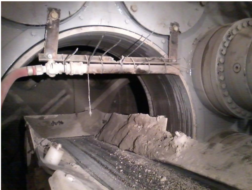
The dust suppression system spraying inside the cutter head.
