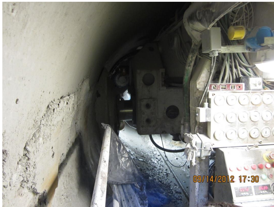
Figure 3.1. The Robbins TBM gripper system.
