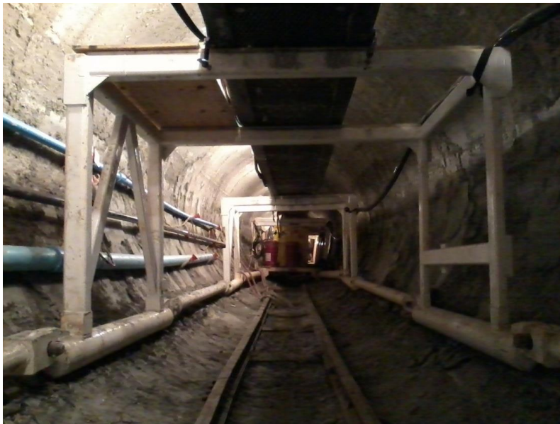
Figure 1.4. Backup system to the TBM. A series of skids will hold the conveyor system up and allow for the muck cars to fit under.
