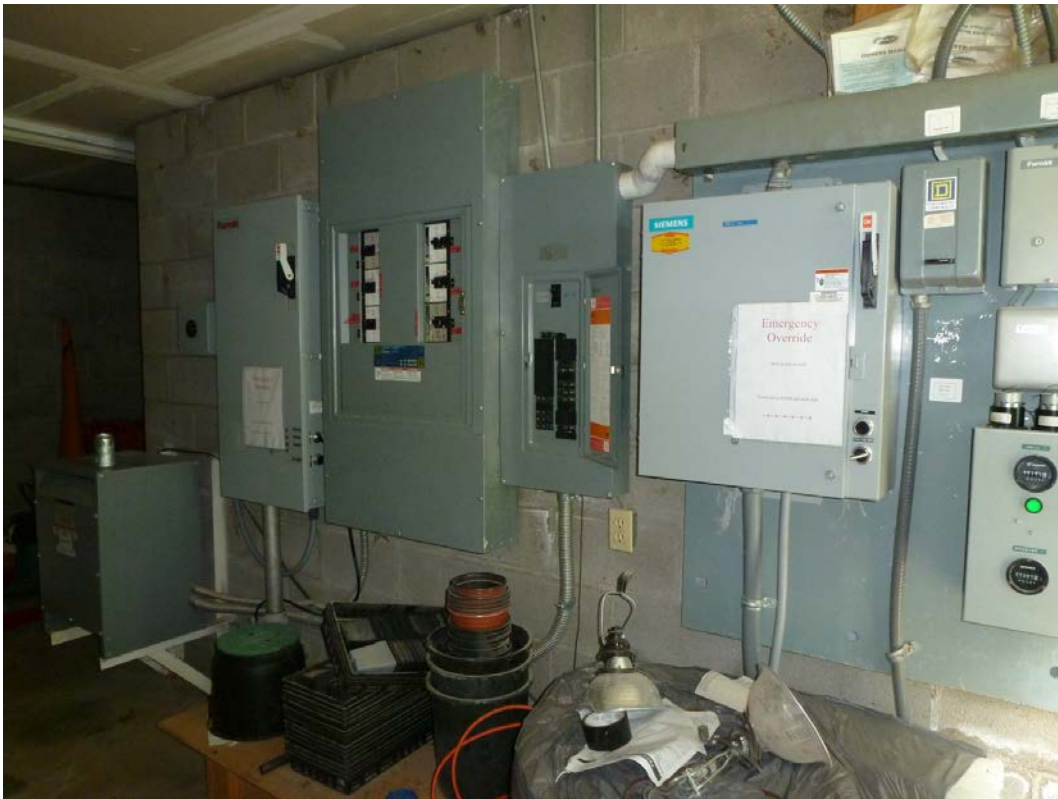
Figure 23: Electrical distribution panels for the residential subdivision
