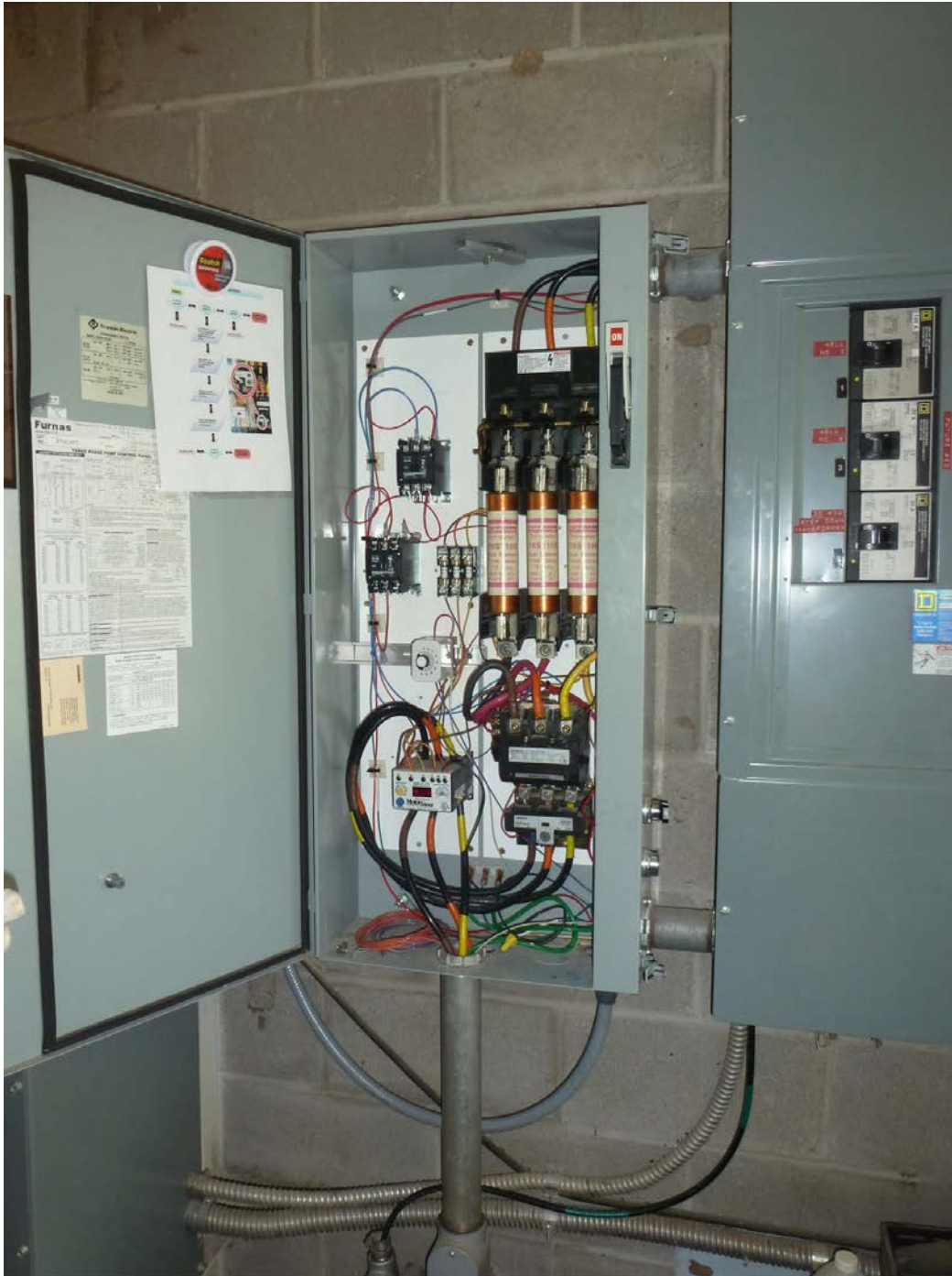
Figure 24: Distribution and motor protection system for the largest motor at the residential subdivision
