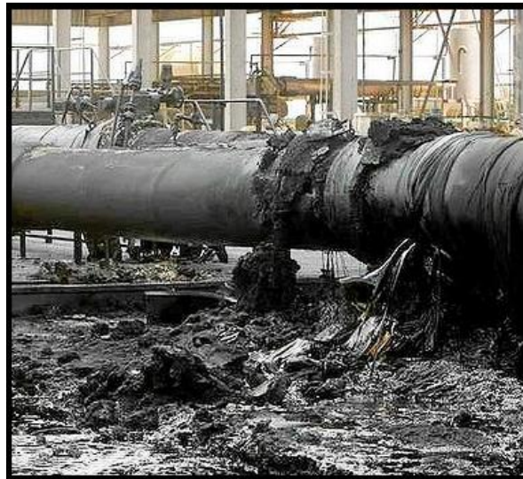
Figure 3-8 Damaged Oil Pipeline. Source: Business Day, February 11, 2013. Web.
