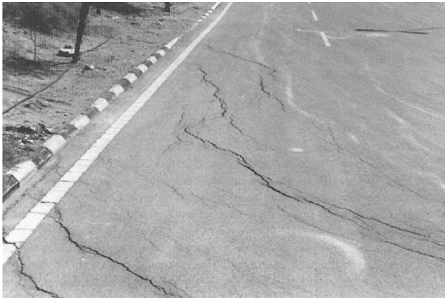
Figure 2.5: Pavement failure (Al Rawas et al., 2005)
