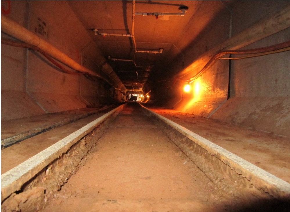
Installed Rails for Bringing out the Dirt and Pipeline for Lubrication as Going Forward
