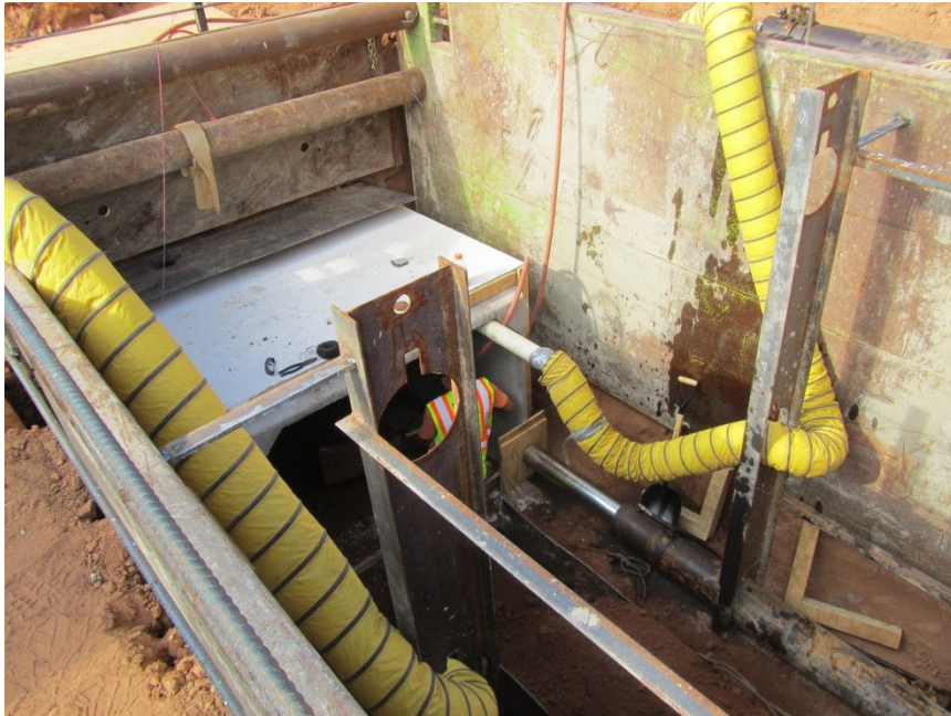
Figure 3.8 Air Supply Lines
