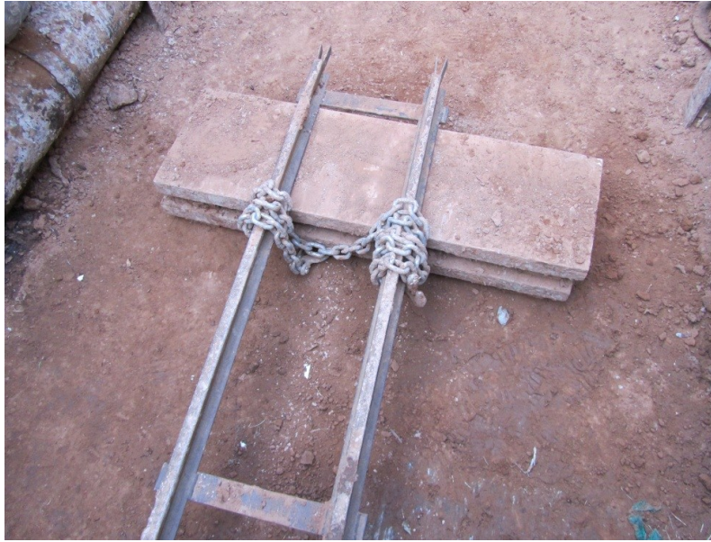
Figure 3.6 Spoil Cart Rail
