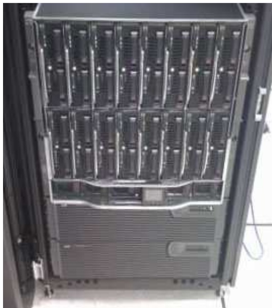
Figure 4 HP blade system C7000 blade enclosure [5]
