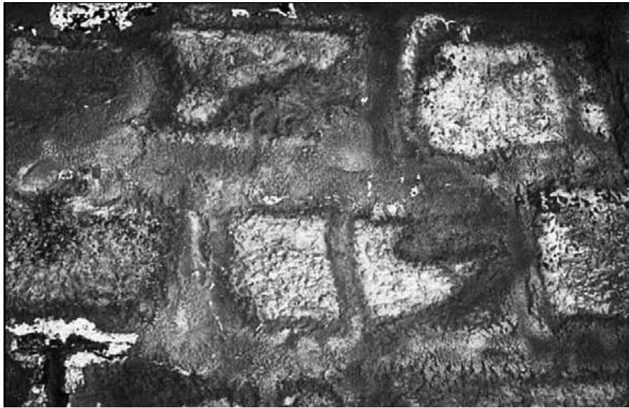
Figure 2.2 Sulfate Induced Heave in Limestone Cladding of Some Slovenian Railway Tunnels (Suput et al. 2003)
