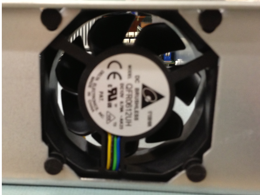
Figure 2.9. Fan installed in Intel Open Compute server.
