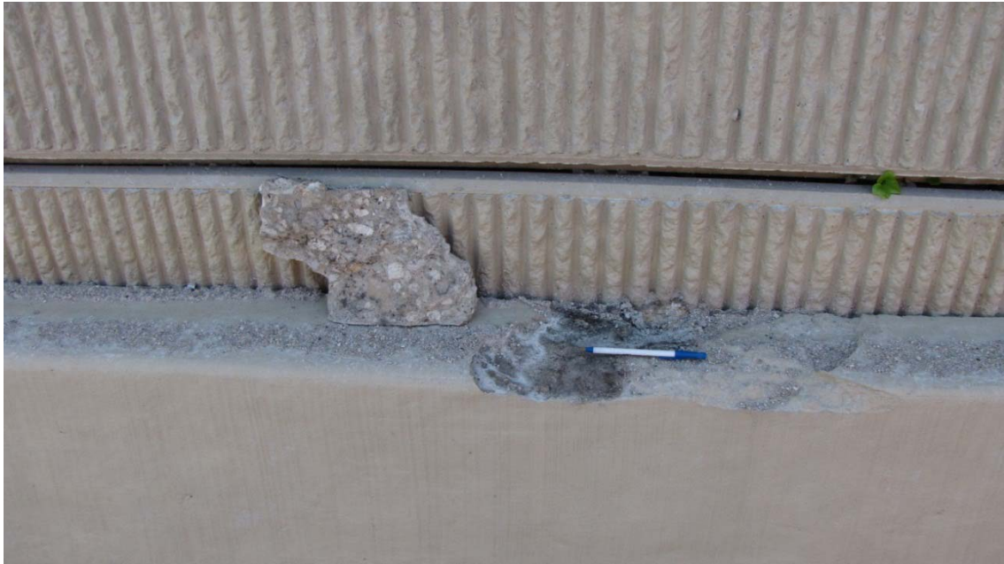
Figure 3-12: Spalled Concrete Traffic Rail at Wall Base
