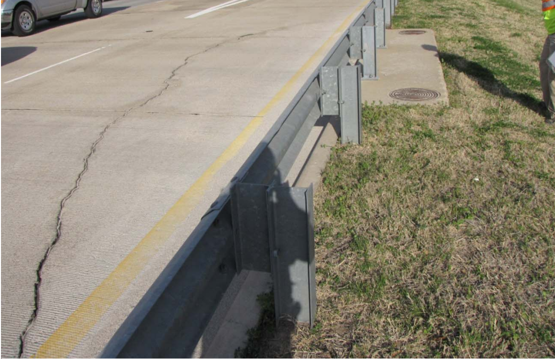
Figure 3-4: Cracking in Retained Zone Pavement
