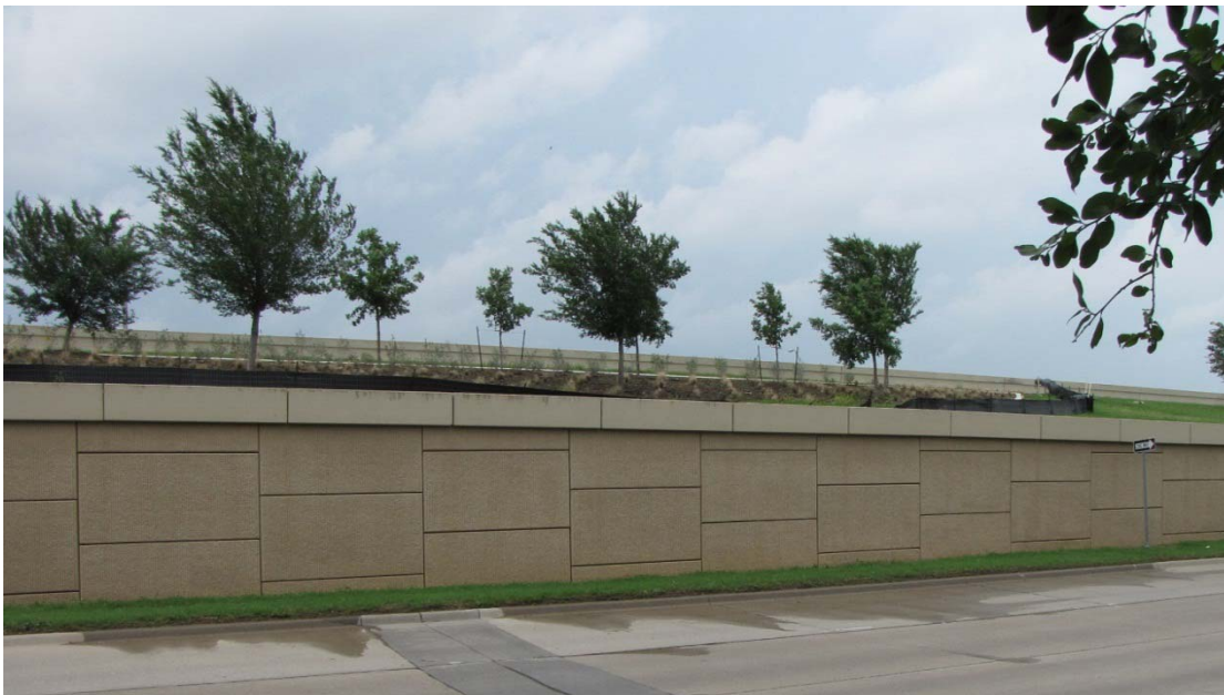
Figure 3-14: Seepage Offset from Base of Wall
