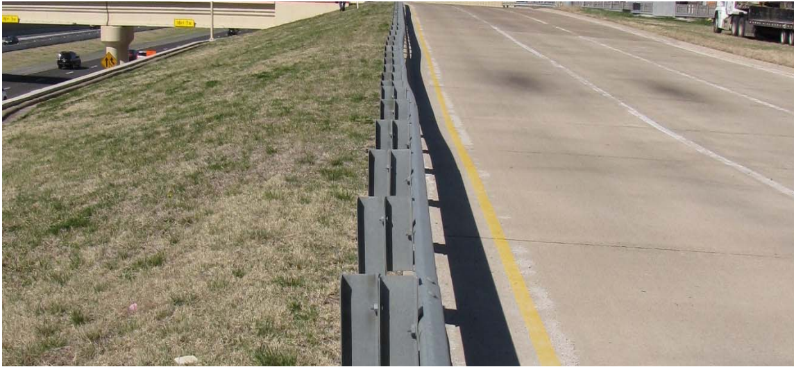
Figure 3-5: Depression in Paving
