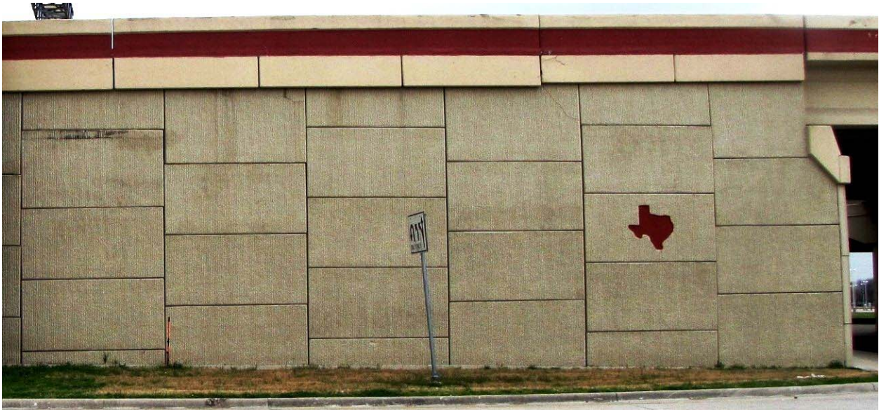
Figure 3-9: Cracked Panels and Coping
