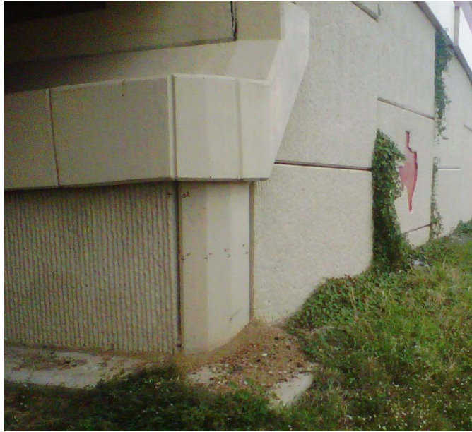
Figure 3-7: Reinforced Zone Material Loss Through Panel Joints
