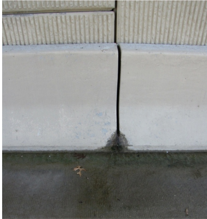
Figure 3-13: Seepage at Base of Wall (through ~3ft tall traffic rail)
