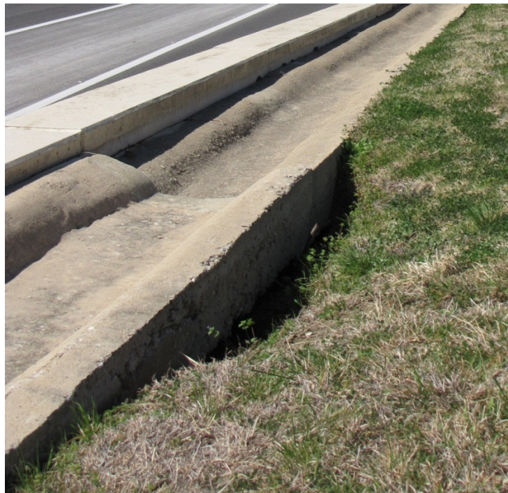
Figure 3-6: Erosion at Adjacent to Wall Flume
