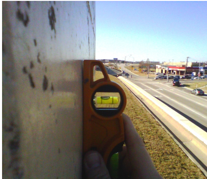
Figure 3-1: Out of Plumb Structure in Retained Zone
