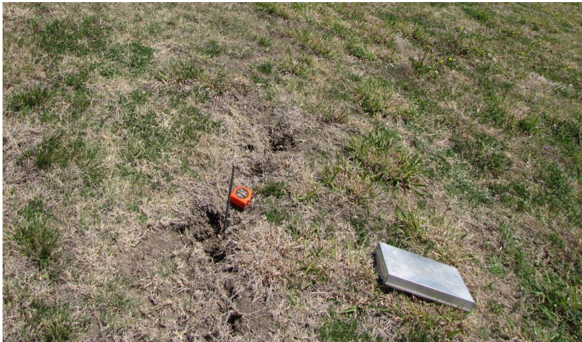
Figure 3-3: Cracking in Retained Zone Soil
