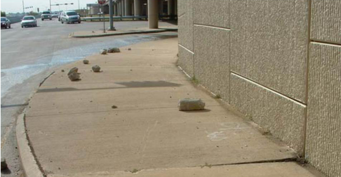
Figure 3-11: Sheared Curb at Wall Base
