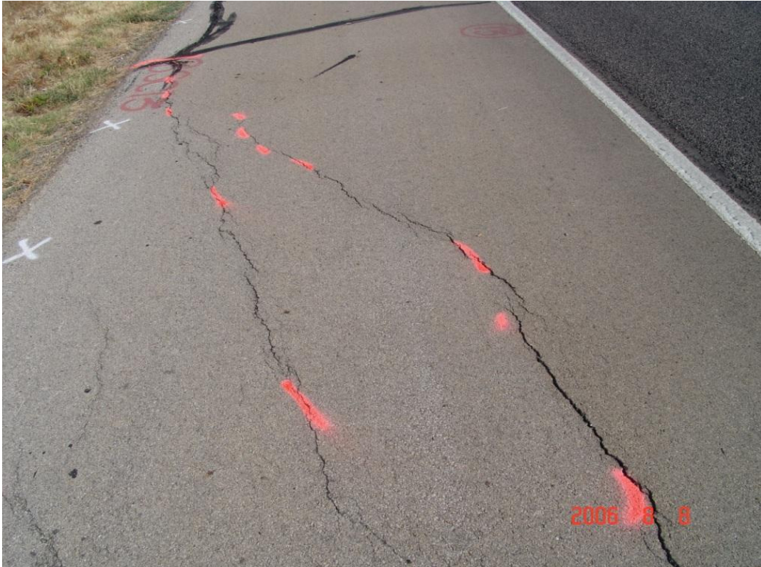
Figure 1-1 Longitudinal and transverse cracks on SH 180
