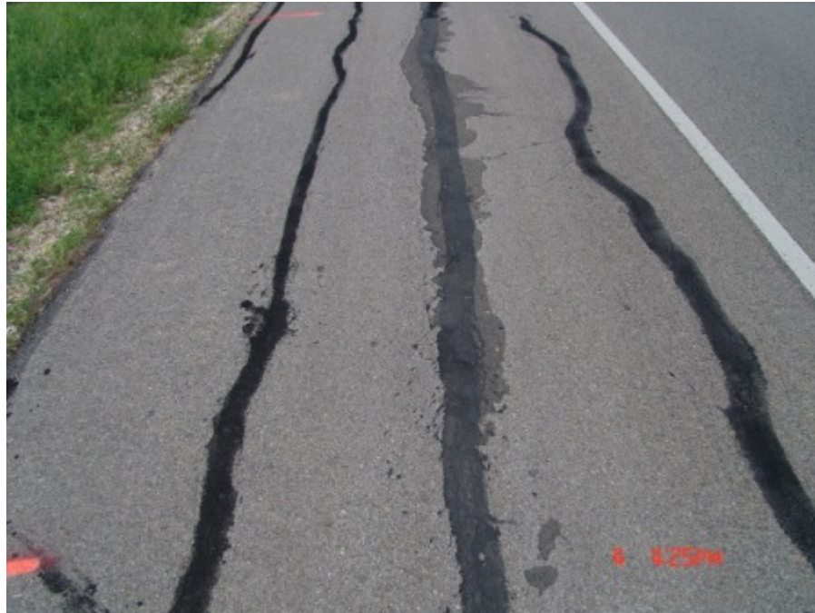
Figure A-45 WC_1 section at Yoakum, TX on April 2007 (Part 1)
