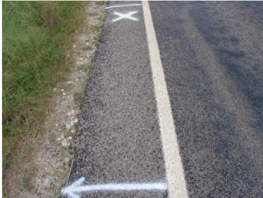
Figure A-107 Control section at Tyler, TX on August 2007 (Part 2)
