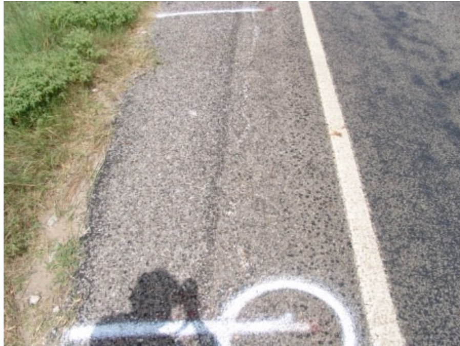
Figure A-109 Control section at Tyler, TX on August 2007 (Part 4)
