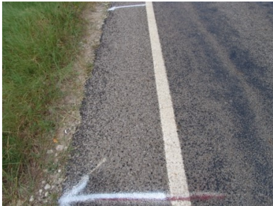
Figure A-106 Control section at Tyler, TX on August 2007 (Part 1)
