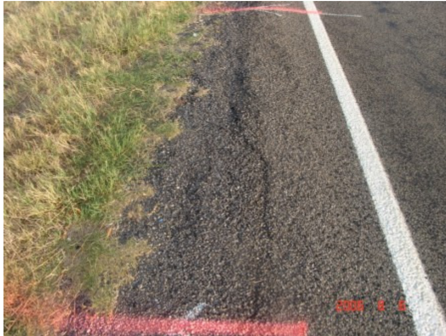
Figure A-79 Control section at Tyler, TX on August 2006 (Part 6)
