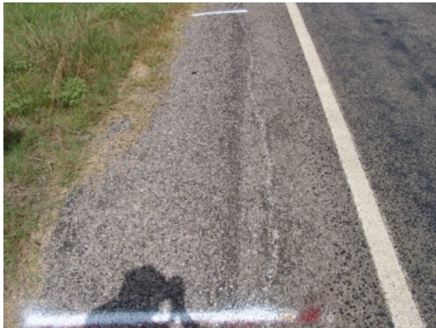
Figure A-110 Control section at Tyler, TX on August 2007 (Part 5)
