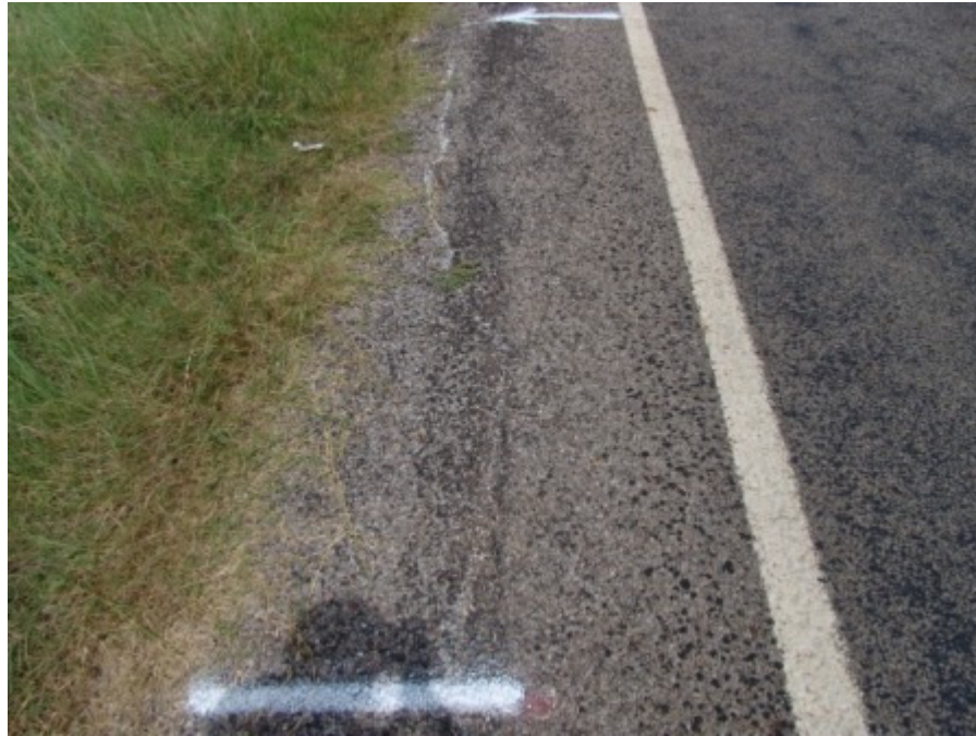
Figure A-111 Control section at Tyler, TX on August 2007 (Part 6)
