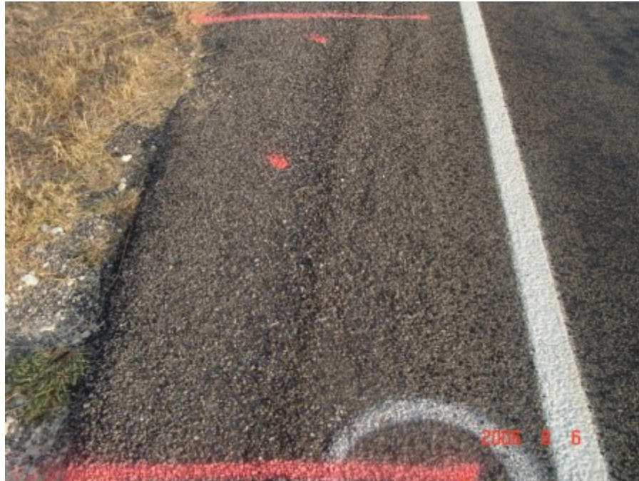
Figure A-77 Control section at Tyler, TX on August 2006 (Part 4)
