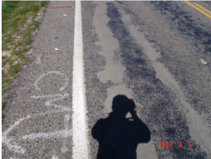
Figure A-81 WC_3 compost treated section at Tyler, TX on March 2007
