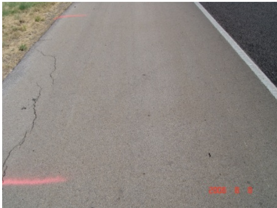
Figure A-2 DMC_1 section at Stephenville, TX on August 2006 (Part 2)
