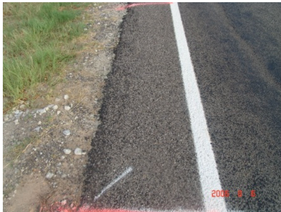
Figure A-74 Control section at Tyler, TX on August 2006 (Part 1)
