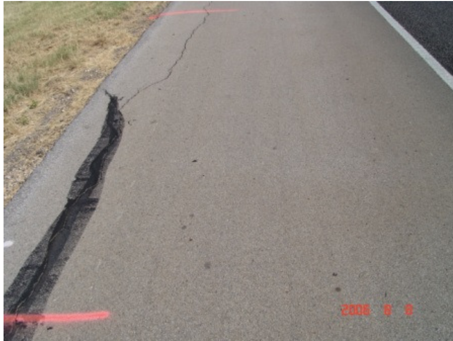
Figure A-1 DMC_1 section at Stephenville, TX on August 2006 (Part 1)
