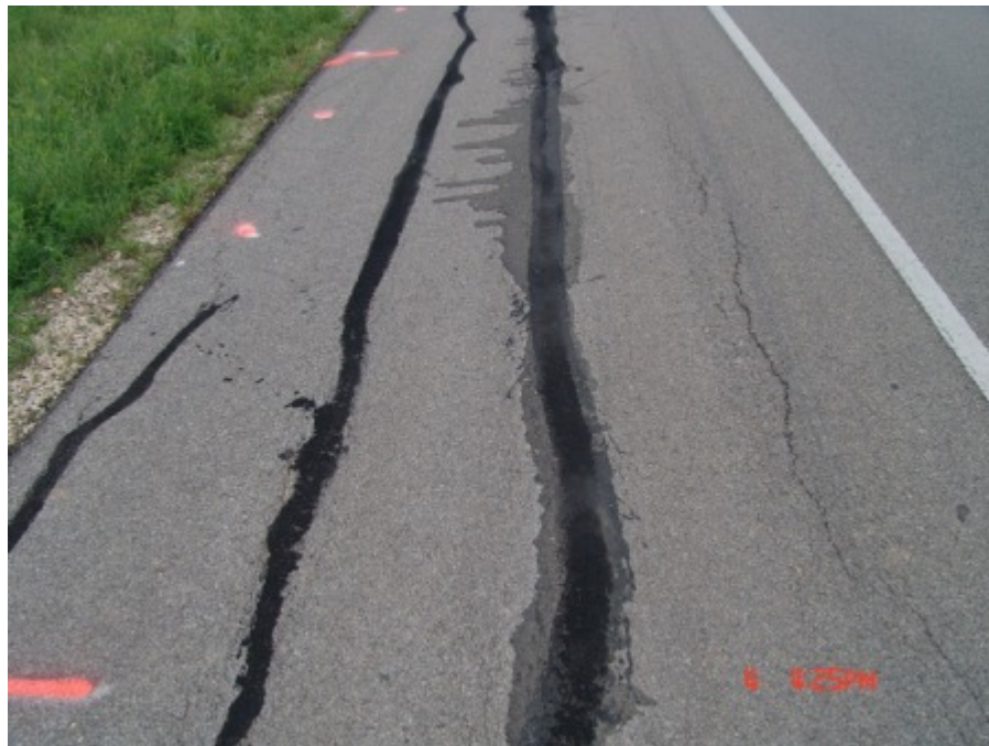
Figure A-46 WC_1 section at Yoakum, TX on April 2007 (Part 2)
