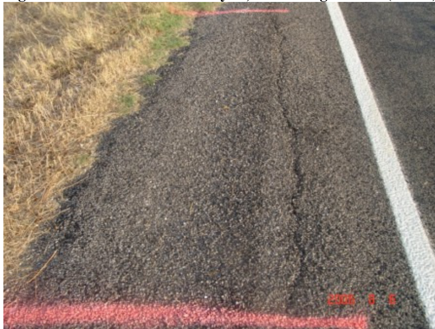
Figure A-78 Control section at Tyler, TX on August 2006 (Part 5)
