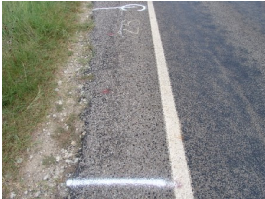
Figure A-108 Control section at Tyler, TX on August 2007 (Part 3)
