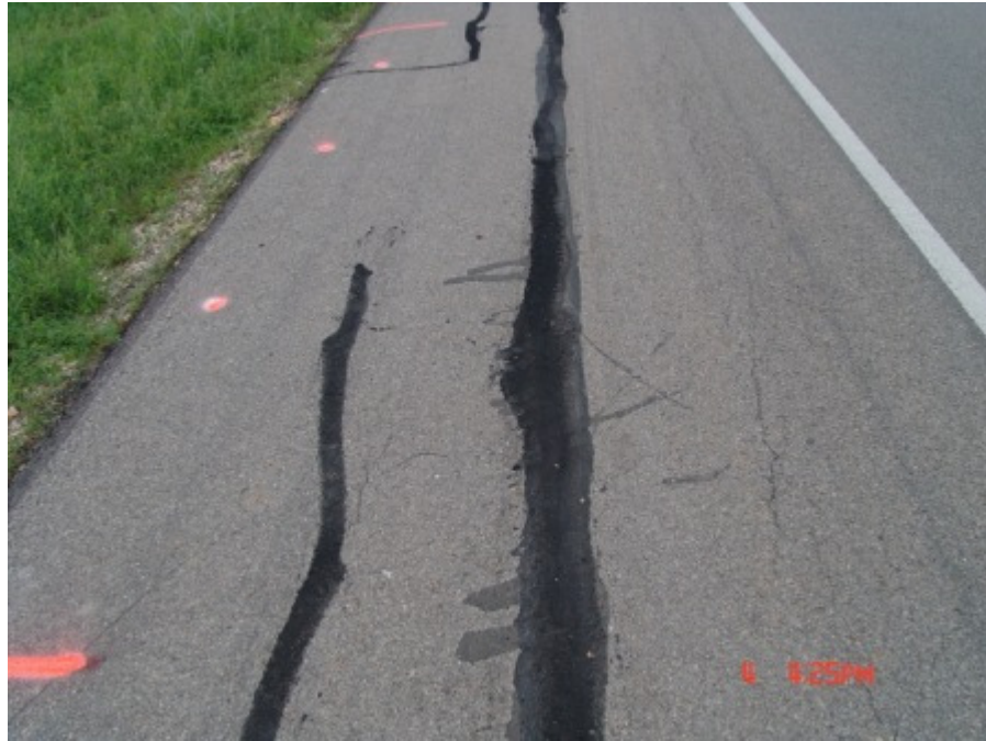
Figure A-47 WC_1 section at Yoakum, TX on April 2007 (Part 3)
