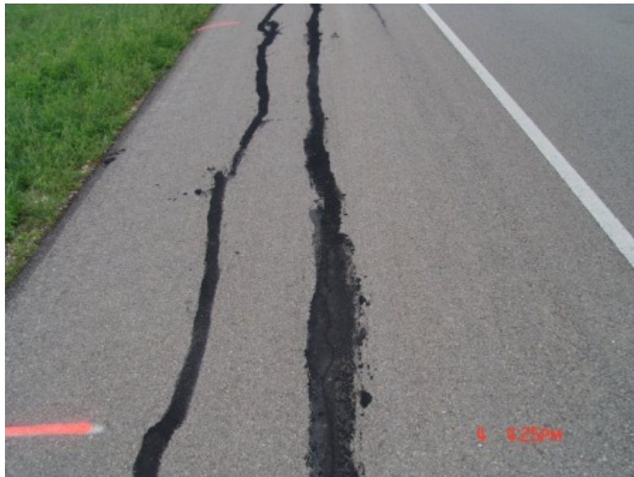
Figure A-48 WC_1 section at Yoakum, TX on April 2007 (Part 4)
