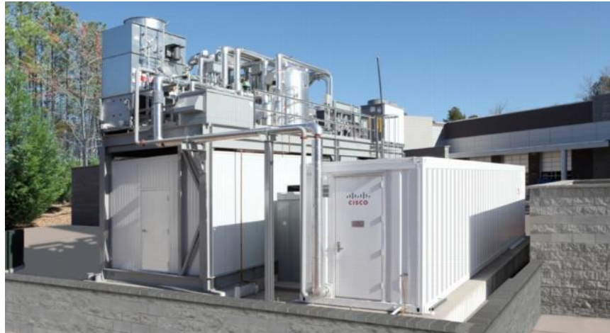
Figure 1.7: Cisco Containerized Data Center [13]
