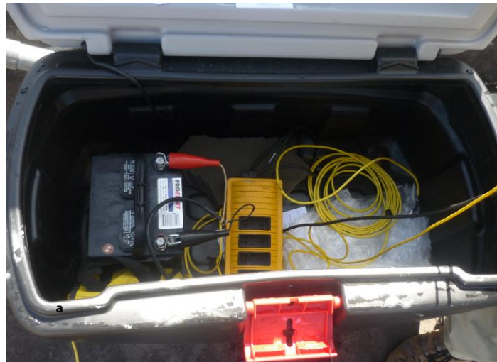
Figure 2.1 Power generating source used on a campaign site - AC power and DC backup.
