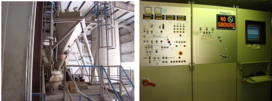
Figure 3.4 Concrete Mixing Facilities in Local Precast Plan
