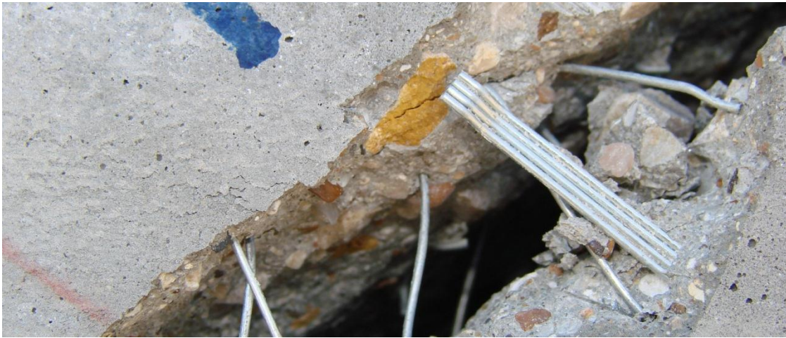
Figure 3.22 Example Photo of Glued Fiber (Remaining Intact)
