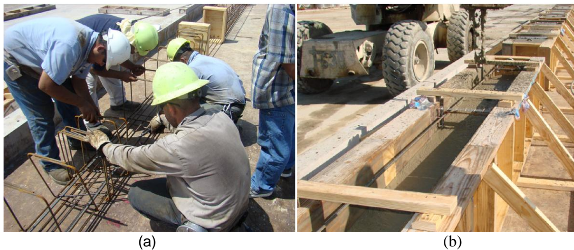
Figure 5.54 Construction of Specimens (a) Preparation of the Steel Cage for PC#2-1(b) Concrete Pouring for SFRPC#2-2
