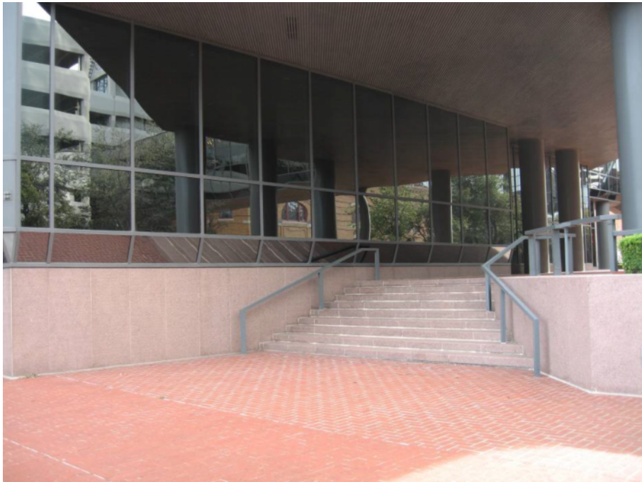
Figure 4.19 Stairs and Handrails Skated in a Commercial Environment (Block 52)
