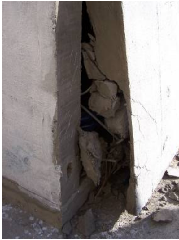
Figure D.14 Lower Left Corner of West Wall
