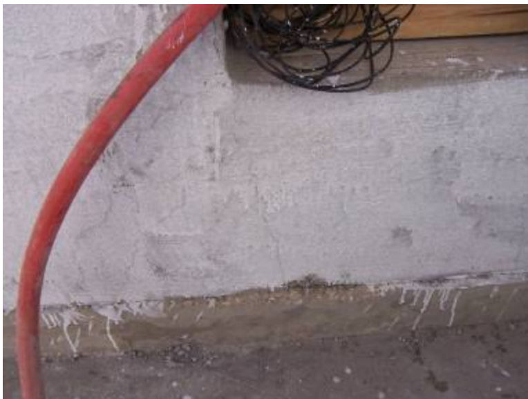
Figure D.2 Cracks at Door before Testing
