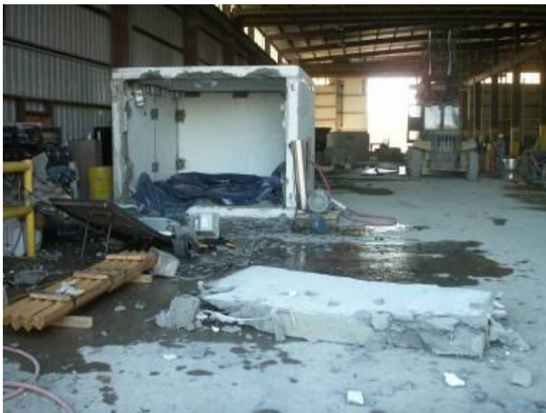
Figure B.4 Left Half of Broken Wall
