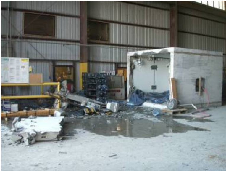
Figure B.3 Failure of Wall
