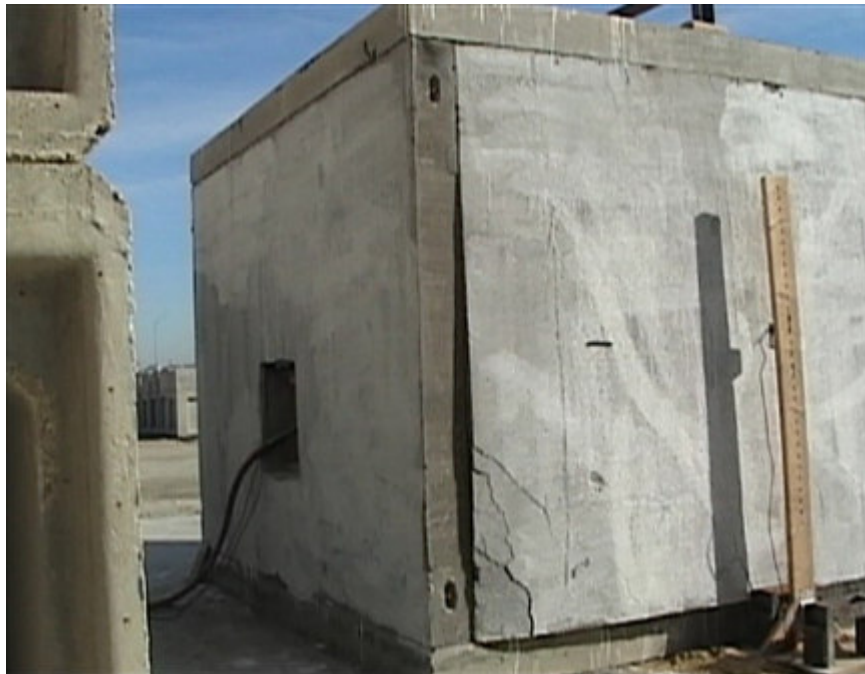
Figure 4.13 Failure of Wall Sequence 1
