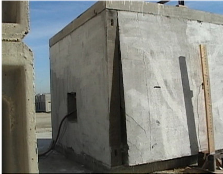
Figure 4.14 Failure of Wall Sequence 2
