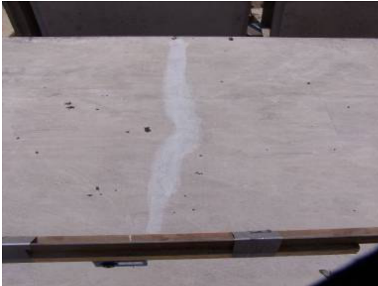
Figure D.3 Crack at Roof before Testing
