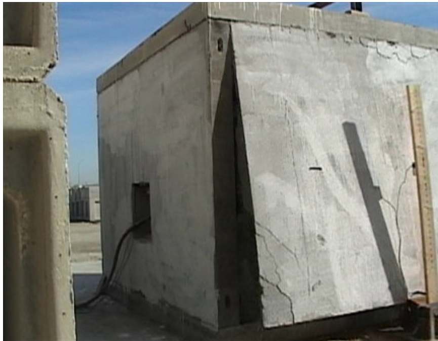
Figure 4.15 Failure of Wall Sequence 3
