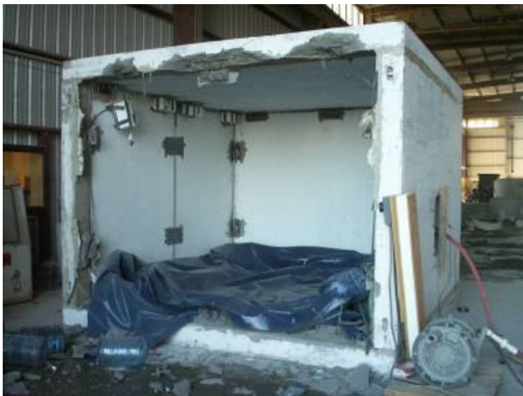
Figure B.2 Failure of Wall
