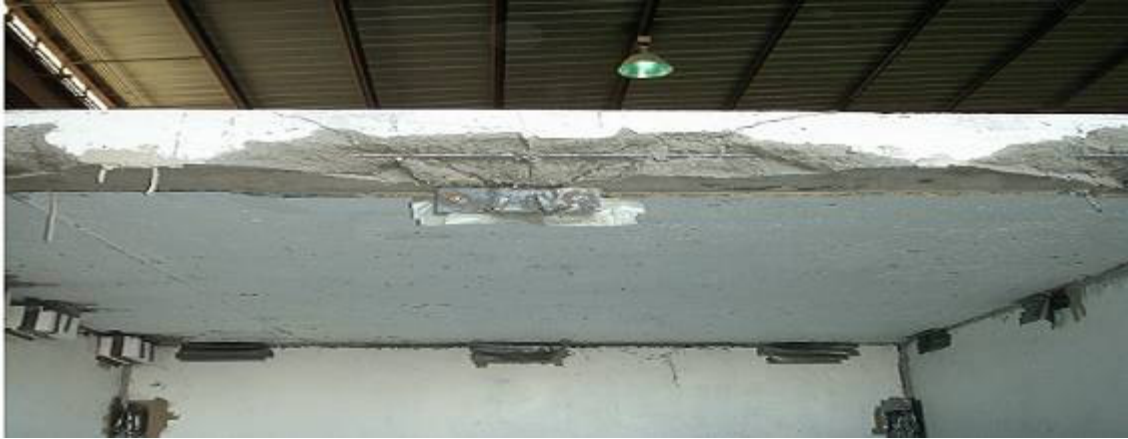
Figure 4.6 Failure at Roof Slab
