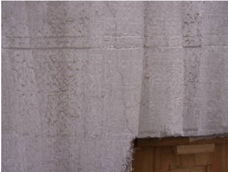
Figure D.1 Cracks at Door before Testing
