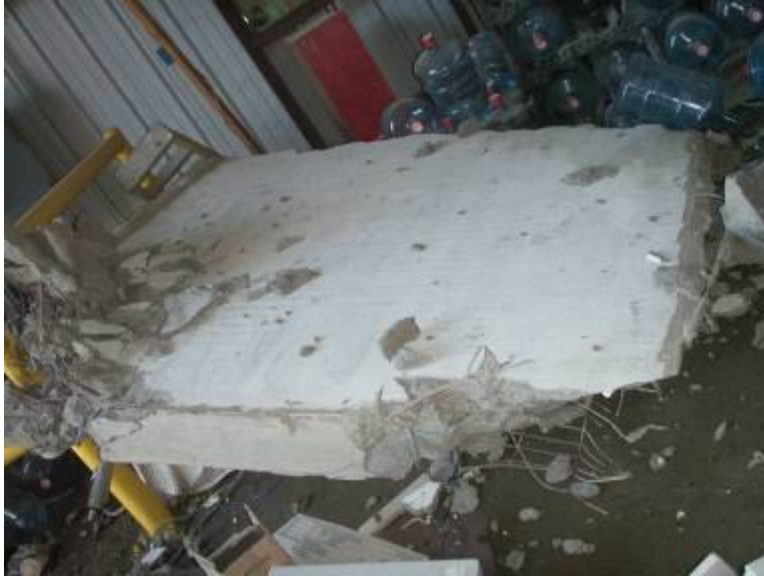
Figure B.5 Right Half of Broken Wall
