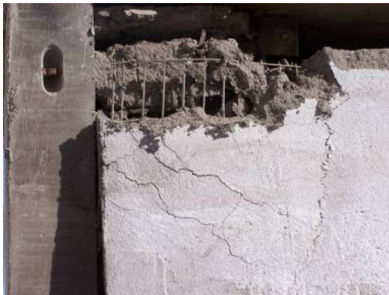
Figure D.7 Left Upper Corner of West Wall
