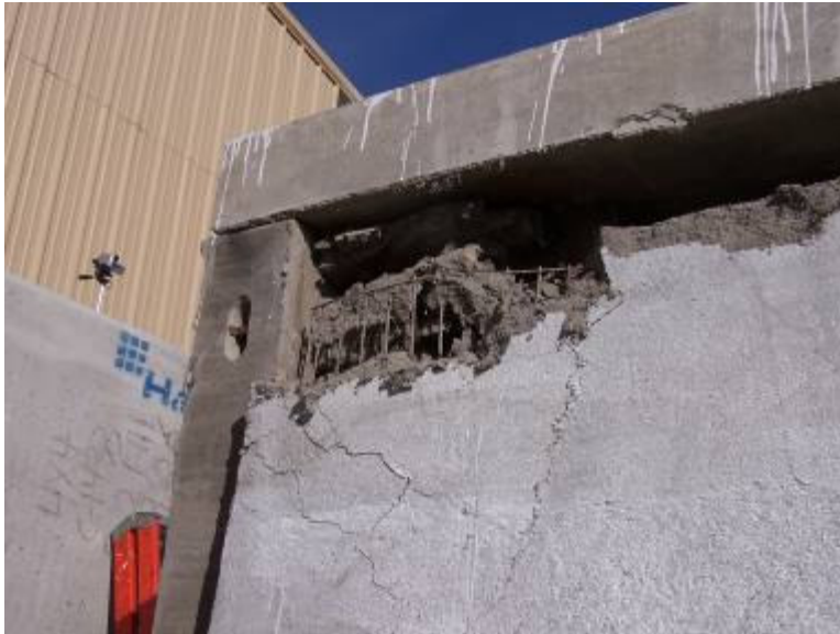
Figure D.12 Failure of Wall Panel
