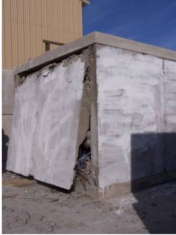
Figure D.5 Failure at West Wall
